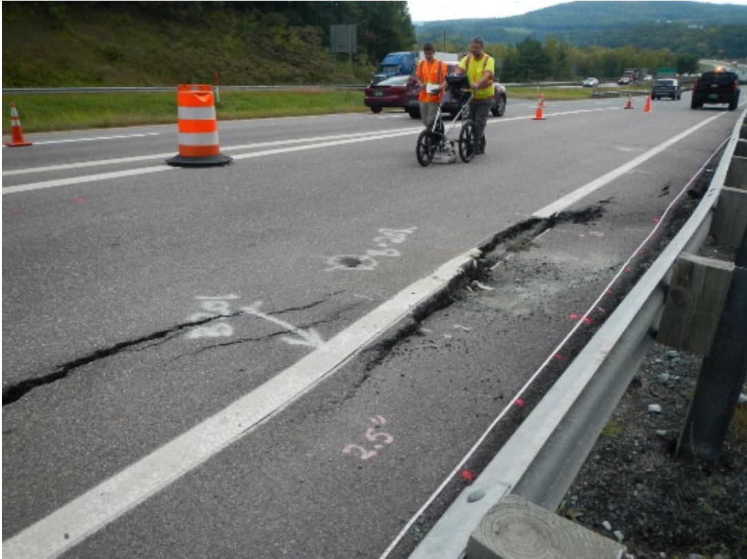
Performed subsurface borings and utilized specialty consultant to perform GPR on area of concern on I-89 in Hartford
