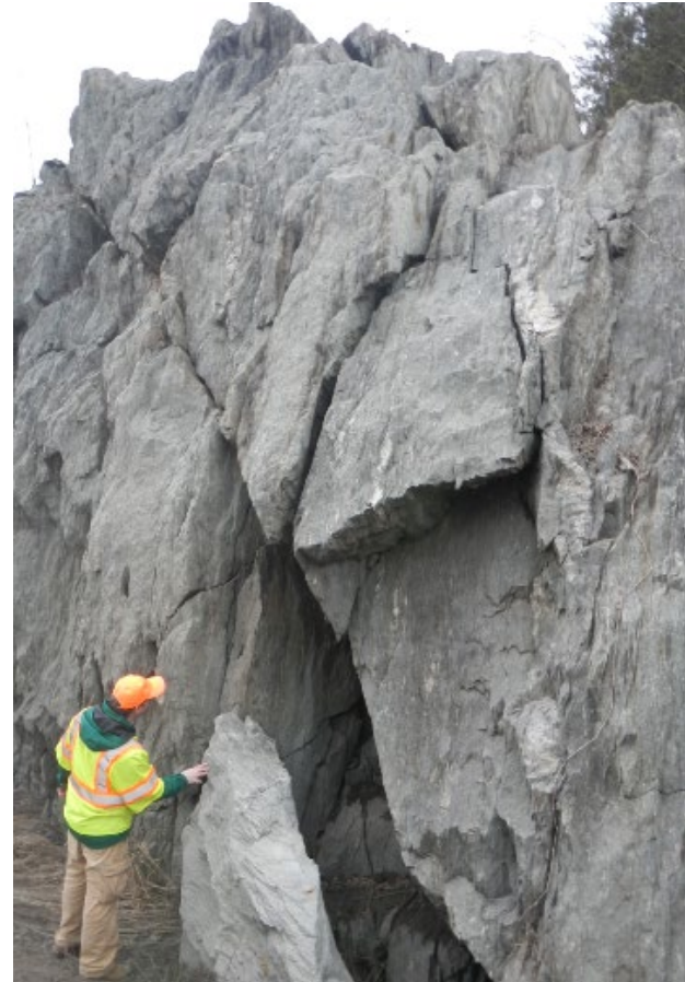
Small rockfall on I-89 in Waterbury
