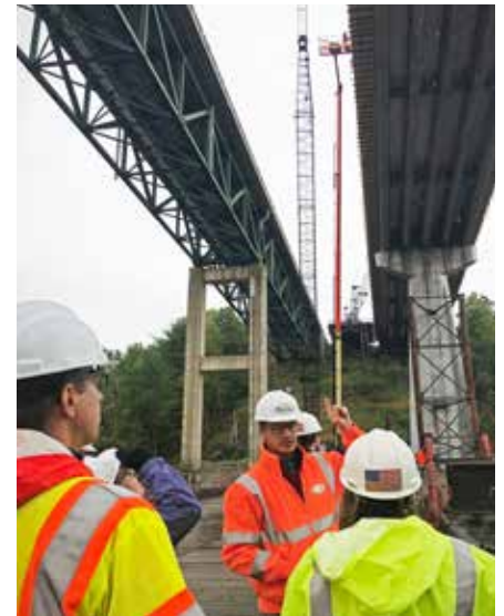
ROCKINGHAM. Replacement of Bridges #24 N&S on I-91 over the Williams River. The multi-year project will create wider bridges and employ precast concrete girders in lieu of the previous steel deck trusses, resulting in longer bridge life.
