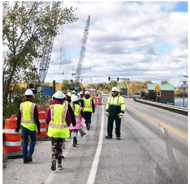
NORTH HERO. The North Hero – Grand Isle Bridge on US RT 2 is a $70 million drawbridge replacement project scheduled for completion in the fall of 2021.
