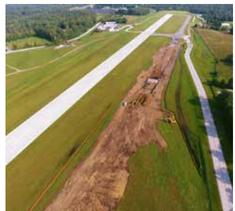
RUTLAND. Construction on the new Taxiway Alpha ("A") at Rutland Southern Vermont Regional Airport. The project will improve safety for aircraft and vehicles that operate at the airport and will make the airport more user-friendly for pilots.
