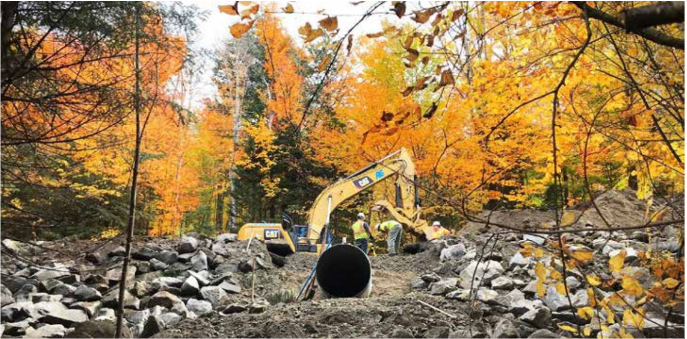
NORTON. Often, VTrans Maintenance Crews work closely with contractors on specific projects. Multiple garage crews assisted in the installation of a 31-foot pipe along VT-114 in Warren's Gore.
