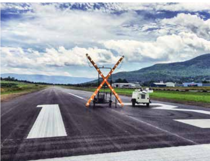
BENNINGTON. A look down a newly extended runway at William H. Morse State Airport.
