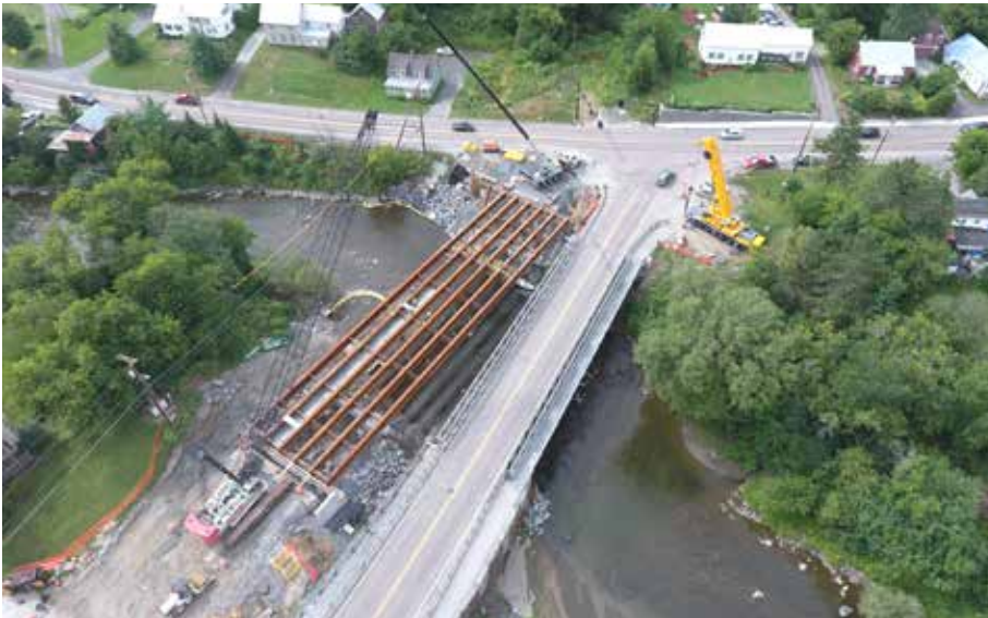
EAST MONTPELIER. Spanning the Winooski River, the original two-span steel VT 14 Bridge along US-2 was replaced with a new 3-lane bridge. Replacing the bridge was a complex project due to the high traffic volumes and the potential impacts on local residents and businesses. A temporary bridge was installed to manage traffic flows while the new bridge was constructed. Through advanced construction methods, the contractor was able to finish ahead of schedule and the new VT 14 Bridge was opened to the public in mid-November.
