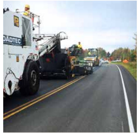
ENOSBURGH. Crews work on a complete resurfacing of VT-105 from Enosburgh Village to Richford.
