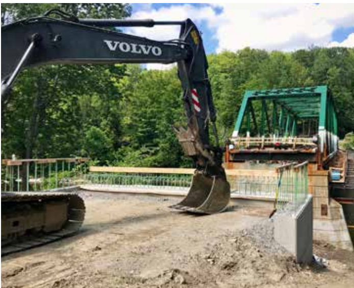
RICHFORD. A multi-year rehabilitation of the Richford-Sutton Bridge along VT-105A over the Missisquoi River.
