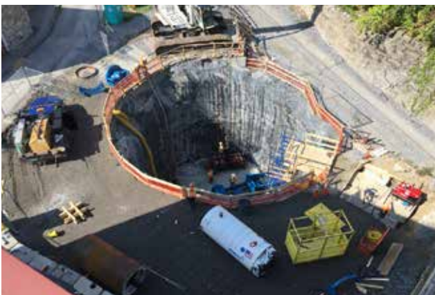
MIDDLEBURY TUNNEL. Replacement of the bridges on VT30 and Merchants Row. $12 million in early work for constructing a complex drainage system was completed in 2018. $45 million is slated for the main project, which is in the final stages of design and will be starting this spring. An expected 10 week rail shutdown is scheduled for summer 2020.
