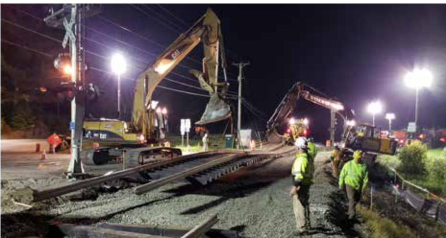
CAVENDISH. This rail construction project involved the replacement of existing railroad crossings with new track along VT 103 in Rutland County.
