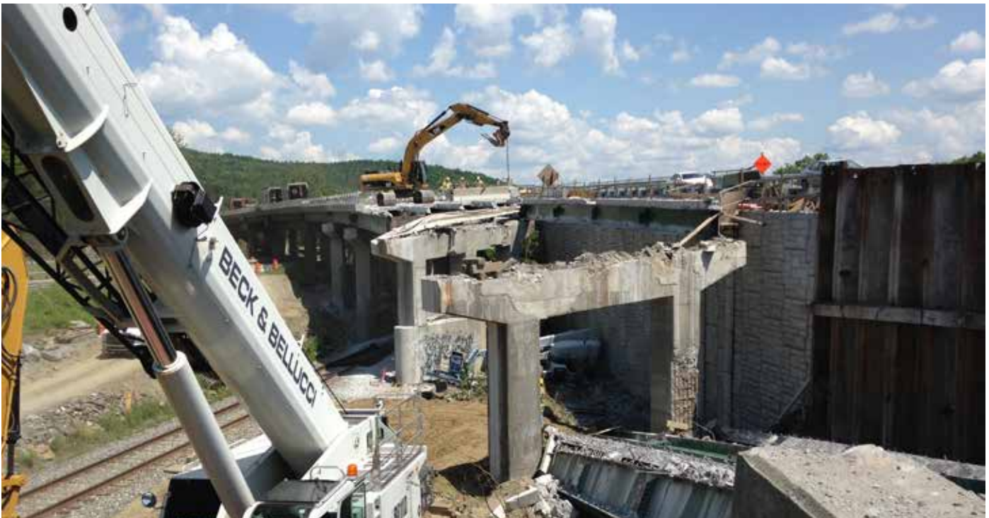
MIDDLESEX. 2018 saw the completion of the US-2 Bridge Replacement project over I-89. Started in 2016, the multi-year project involved the construction of a completely new bridge structure and the demolition of the existing bridge.
