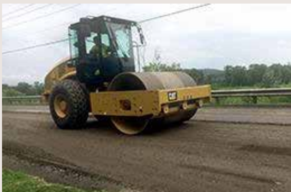
PAVING THE WAY FOR INTELLIGENT COMPACTION IN VERMONT Evaluating Intelligent Compaction data today can pave the way for Vermont's future pavement projects. This research project will provide the Agency with guidelines and recommendations to take advantage of new technology and improve roadway construction.
