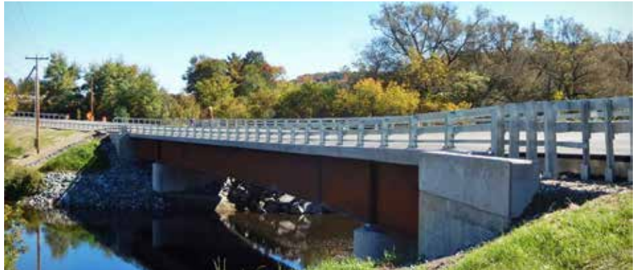
MORRISTOWN. The new VT 15A Bridge over the Lamoille River replaced a decade-old temporary bridge. The new 230-foot bridge features wider lanes and added two 3-foot shoulders for pedestrian crossing.
