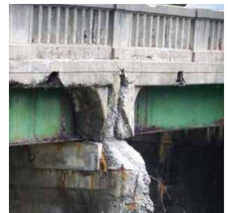
EAST MONTPELIER. Before being replaced, the 80-year-old VT 14 Bridge over the Winooski River was in visibly deteriorating condition and did not meet current design standards. See page 11 to see how the new bridge looks now.
