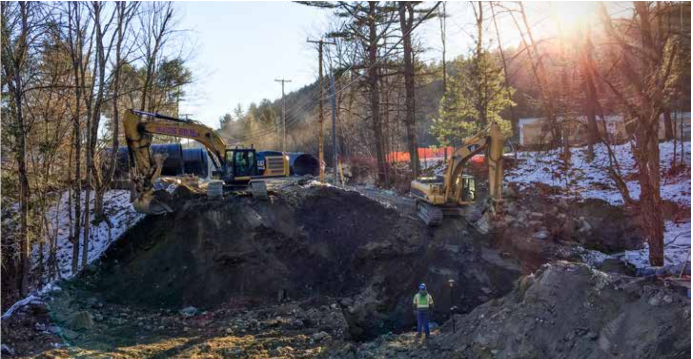
HARTFORD. After a weather event, a backed-up culvert caused significant damage to the subsurface roadway along US-5. Crews worked diligently through cold weather to replace the major culvert and restore the roadway.
