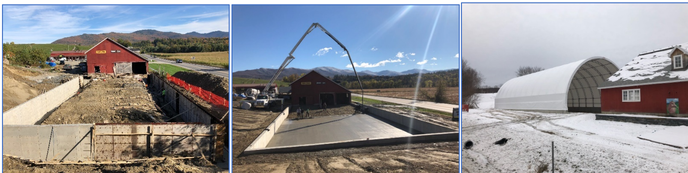
From left to right, site prep work, concrete wall & slab pour and the finished hoop structure.
