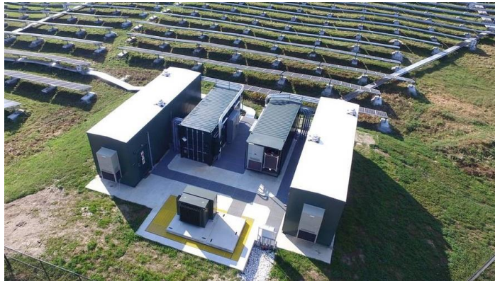
The US' first utility scale solar plus storage Installation (Vermont)
