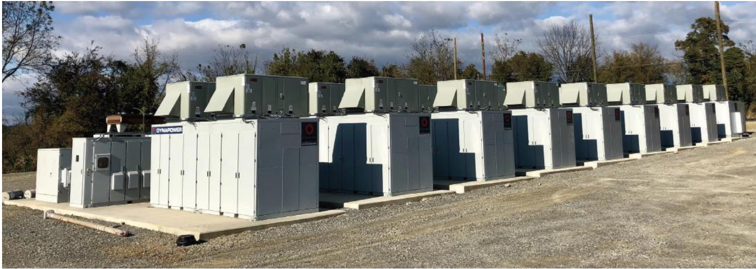
DYNAPOWER 20MW/20MWh installation in New Jersey
