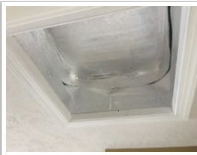
Air leakage at attic hatch and typical solution:
