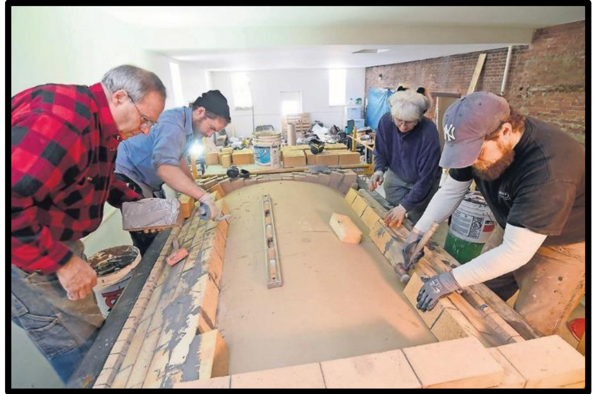
Rebuilding of the wood-fired oven in the historic Rise Up Bakery adjacent to the Old Labor Hall in Barre
