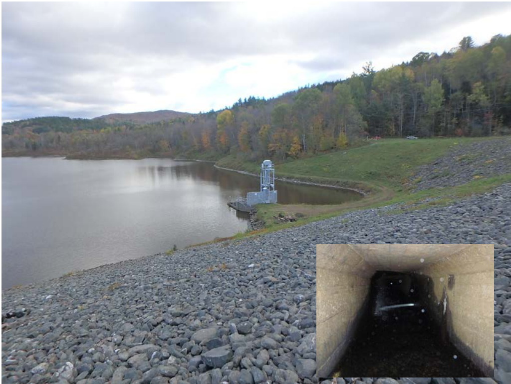
Wrightsville Dam, principal spillway intake structure and leak in spillway tunnel
