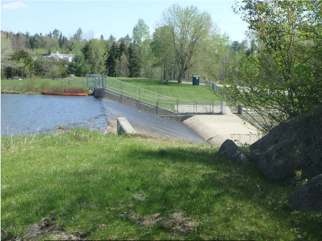
Miles Pond Dam, various minor repairs needed.
