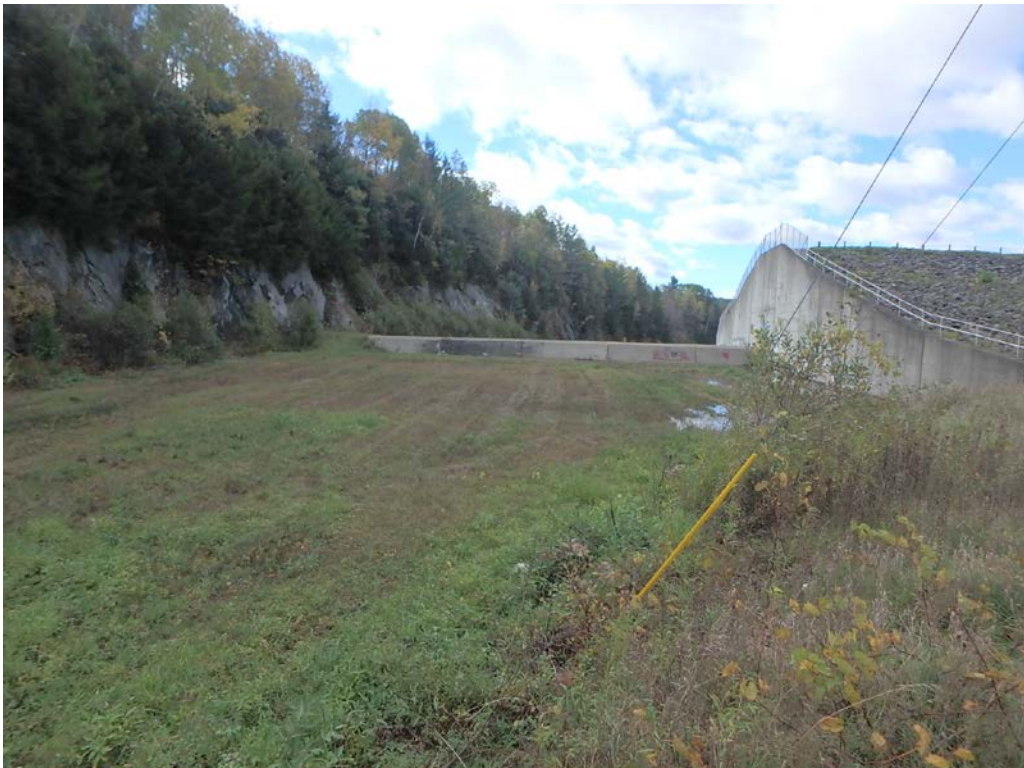
Wrightsville Dam, aux. spillway, note overgrown and aging rock cut at left side of image
