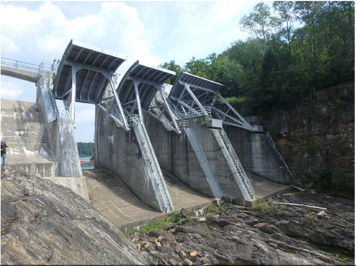
Waterbury Dam Spillway, the access ladders requiring a fall protection system can be seen.
