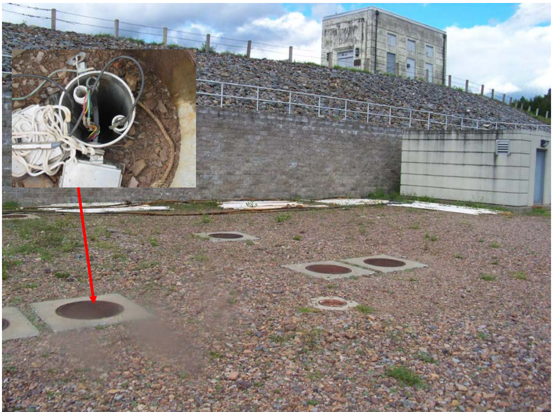
Waterbury Dam Seepage Collection System
