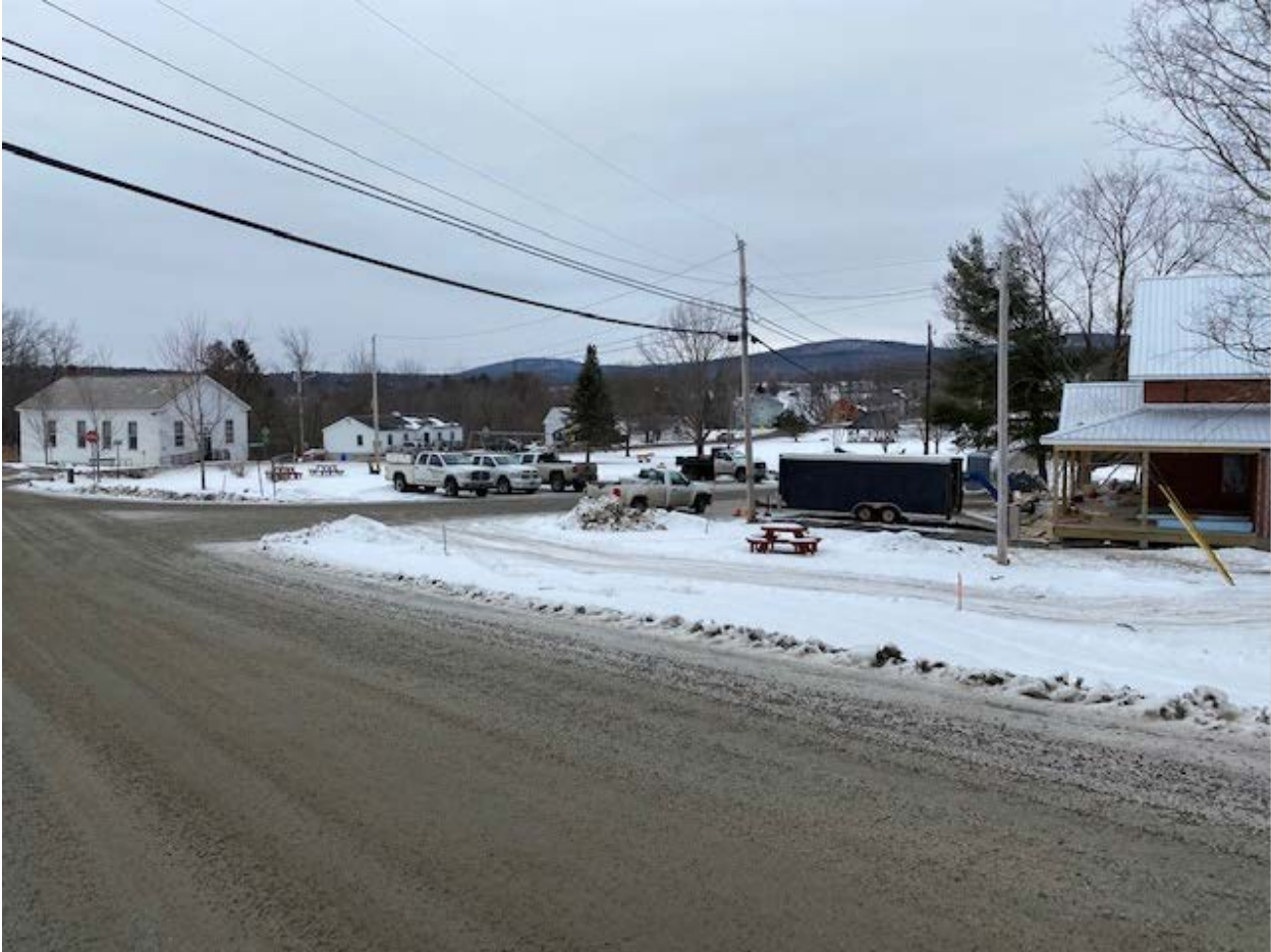
Parcel 2 new Westford County Store & Cafe under construction. Town Common, Public Library, Town Office & Parcel 1 in background. (view north)
