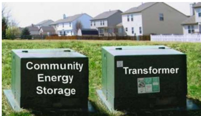
Source: American Electric Power (AEP)
