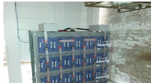
PowerGuru 32 kWh battery install in Pownal
