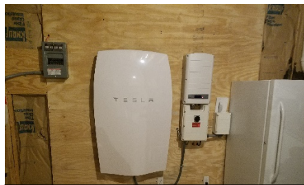
Tesla Powerwall unit installed by Peck Electric in S. Burlington.
