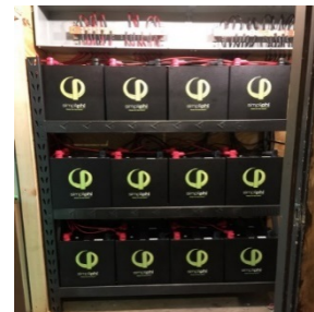
Simpliphi system at Emerald Lake
