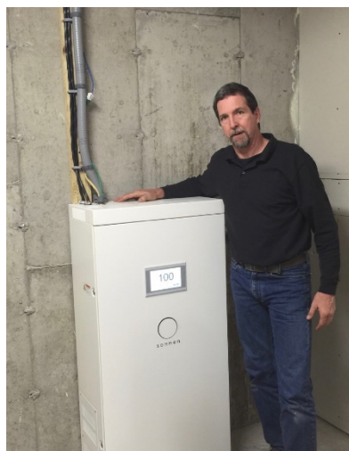
Bill Laberge of Grassroots Solar with a Sonnenbatterie
