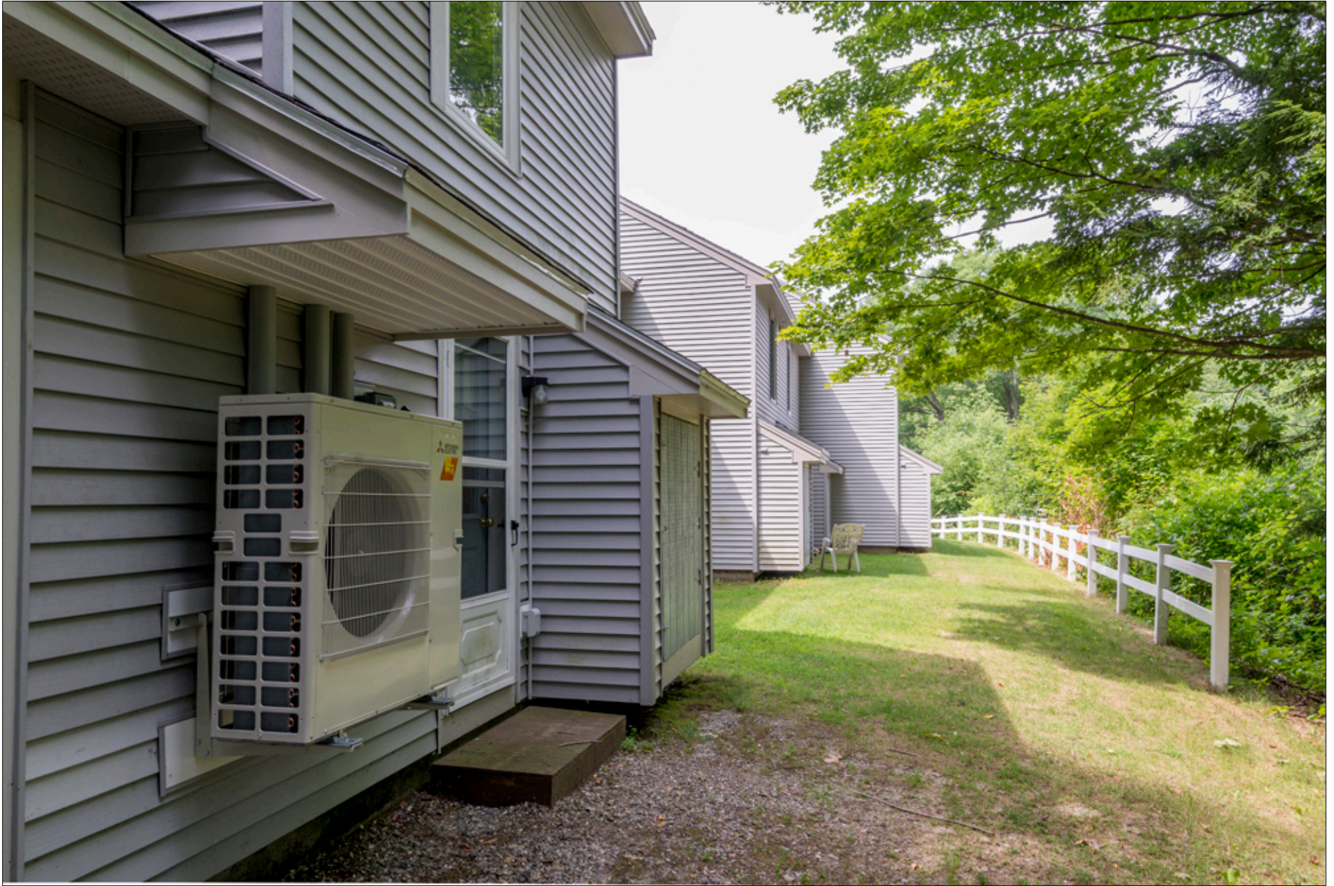
New heat pumps installed as part of a pilot program
