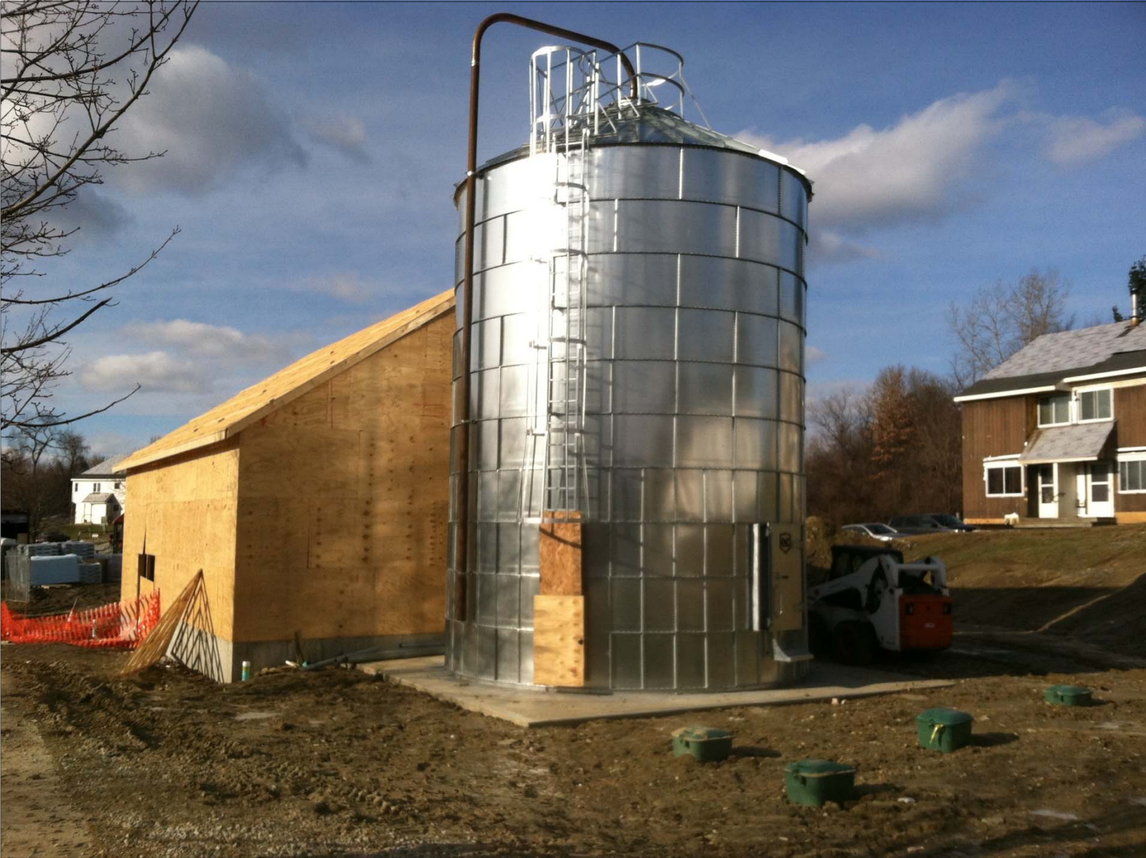
The new silo and central biomass heating system building is under construction.
