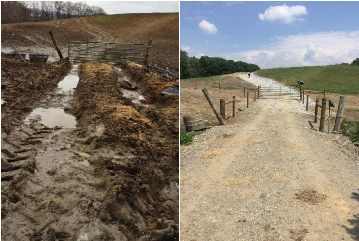
Figure 21. Before (left) and after (right) installation of livestock exclusion fencing and improved laneway and water crossing, completed by Poultney Mettowee Conservation District with ANR funding
