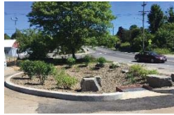
Bioretention system on Center Street, Northfield completed by Central Vermont Regional Planning Commission (see Figure 26)
