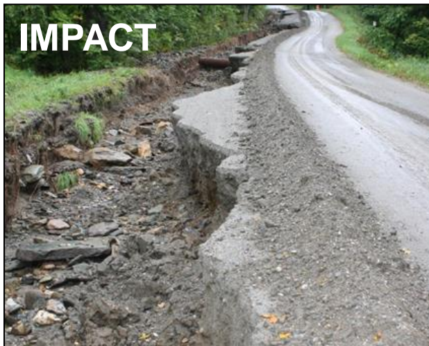
Eroding roadside ditch
