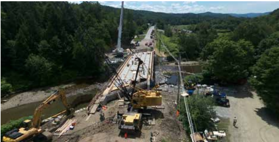
WAITSFIELD. Construction of a replacement bridge over the Mad River along VT100 in Waitsfield. The new bridge is being constructed using Accelerated Bridge Construction methods to minimize the length of the bridge closure.
