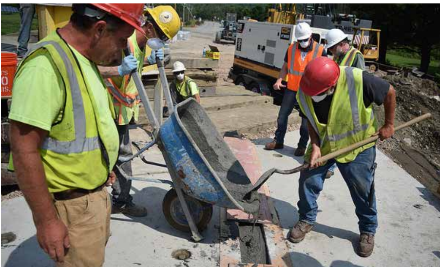
The VT100 bridge project in Waitsfield is the first use of Ultra-High Performance Concrete in Vermont. UHPC provides added resilience over traditional concrete.
