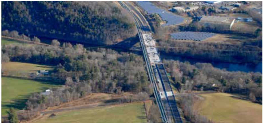
BRATTLEBORO. Two aging steel bridges are being replaced with a single concrete span on I-91.
