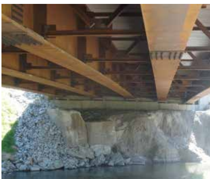
WAITSFIELD. Accelerated bridge construction in Waitsfield utilized innovative approaches by using partial depth deck panels as opposed to full depth panels. These lightweight panels reduced the risk of conflicts during placement and were much easier to lift into place.
