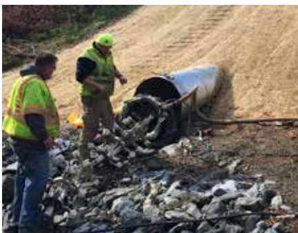
VTrans employees install a culvert liner. Liners are cost effective solutions for prolonging the life of culverts.
