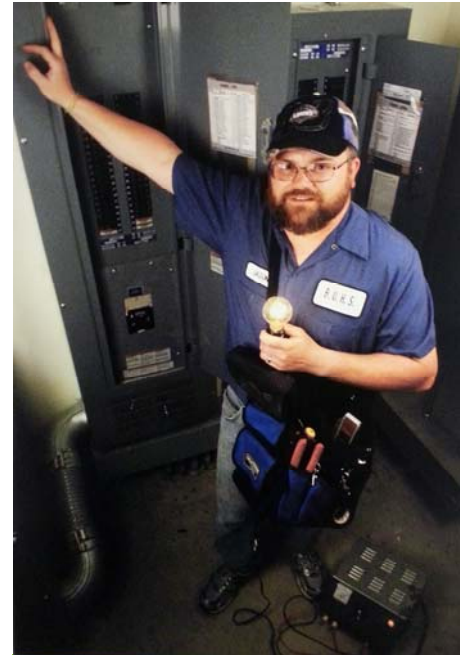
Jason Allbee, a Master Electrician at Brattleboro Union High School, a school that has pledged to reduce energy use.
