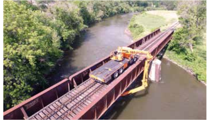
MONTPELIER. VTrans Rail Bridge Inspection Team operating the brand new Aspen Aerials A30 "Snooper" truck at bridge 305 on the Washington County Railroad this Spring.
