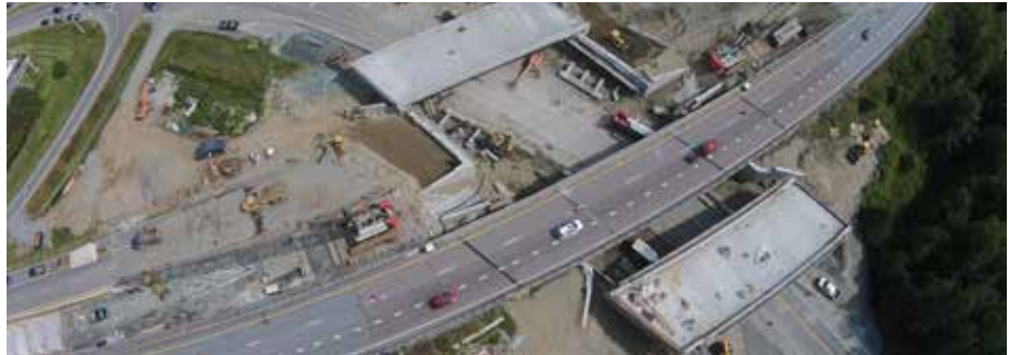
HARTFORD. Using slide-in construction methods, two bridges on I-91 were replaced over two weekends in August.
