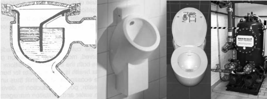
Figure 2 Siphon for waterless urinals invented by Beets, 1885: Oil forms a layer on top of the urine and stops smells (left, Lange, 2002), waterless urinal of GTZ Headquarters (middle, Keramag) and vacuum toilet and pumping station of KfW Building (right, GTZ project data-sheets 2006)
