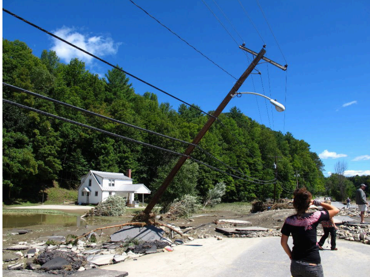
Figure 9: Flooding in Woodstock, VT as a result of Tropical Storm Irene. Photo: Phebe Meyers
