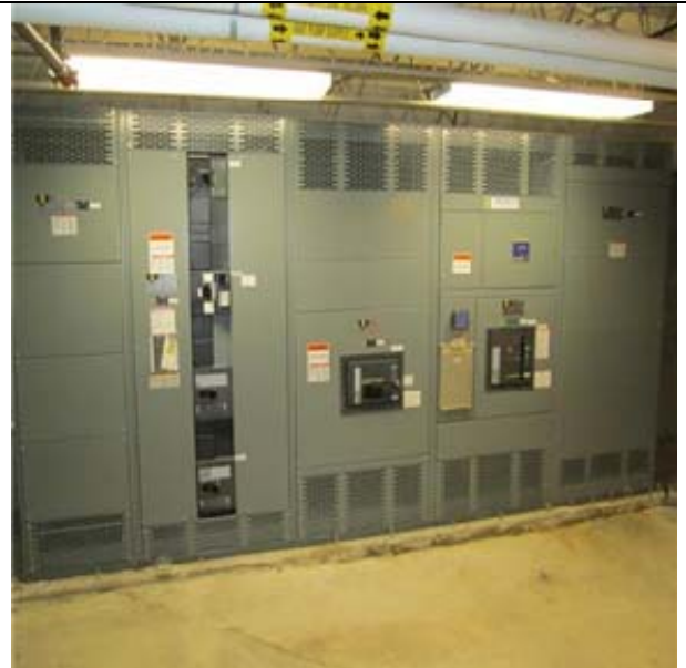
Main electric service switchgear
