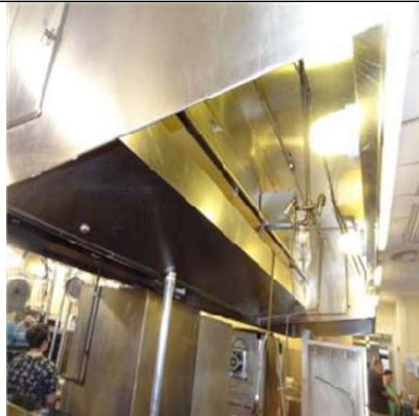
Cook hood with fire suppression
