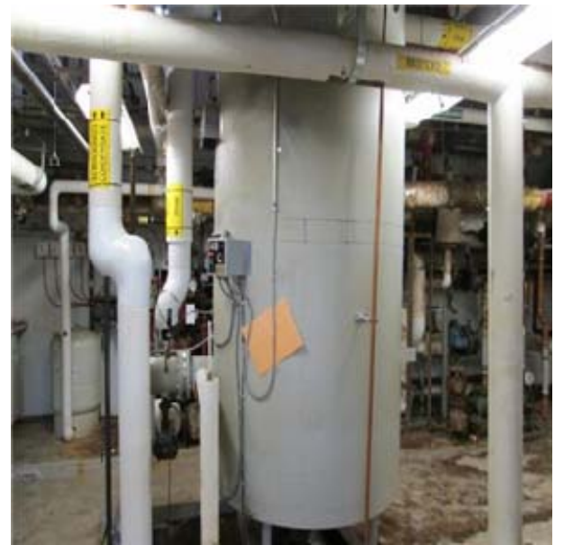
Laundry hot-water steam-fed tank
