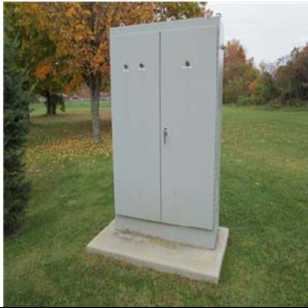
Well pump controller
