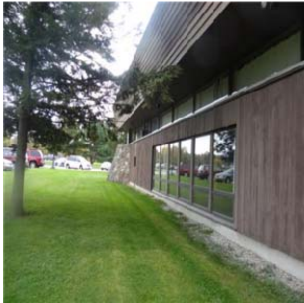
Poor site grading at building perimeters
