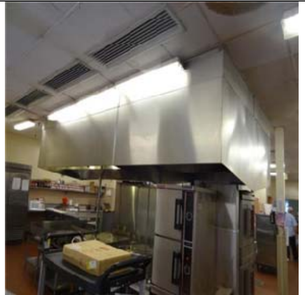
Cook hood with fire suppression
