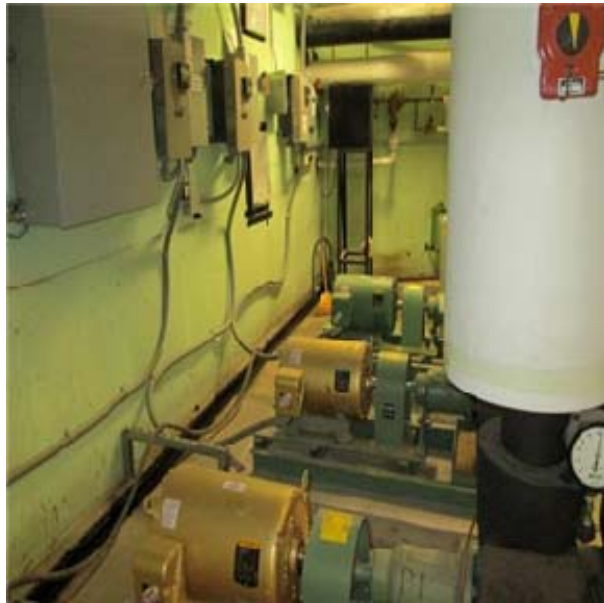
Geothermal system circulation pumps
