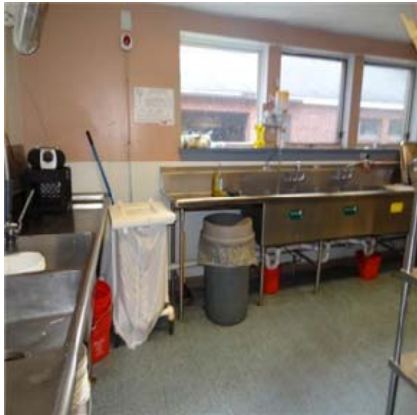
3-compartment sink with drain
