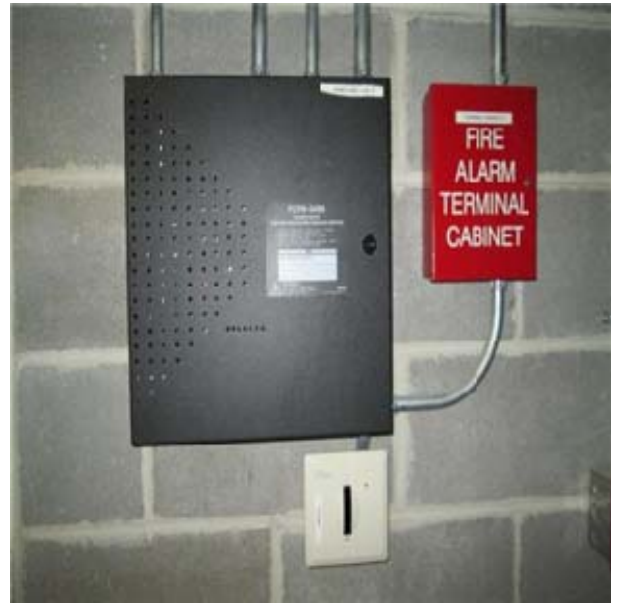
Addressable fire alarm system panel
