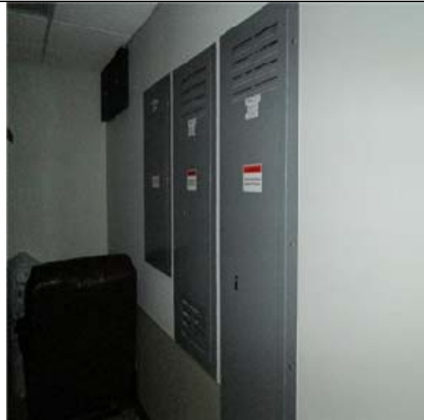
Electrical distribution panels
