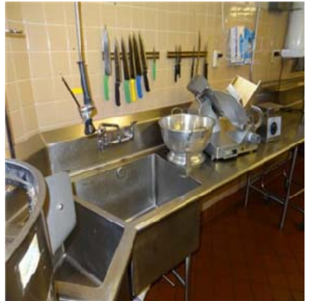
Custom corner sink
