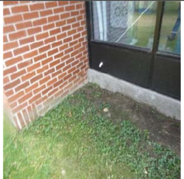
Poor site grading at building perimeter
