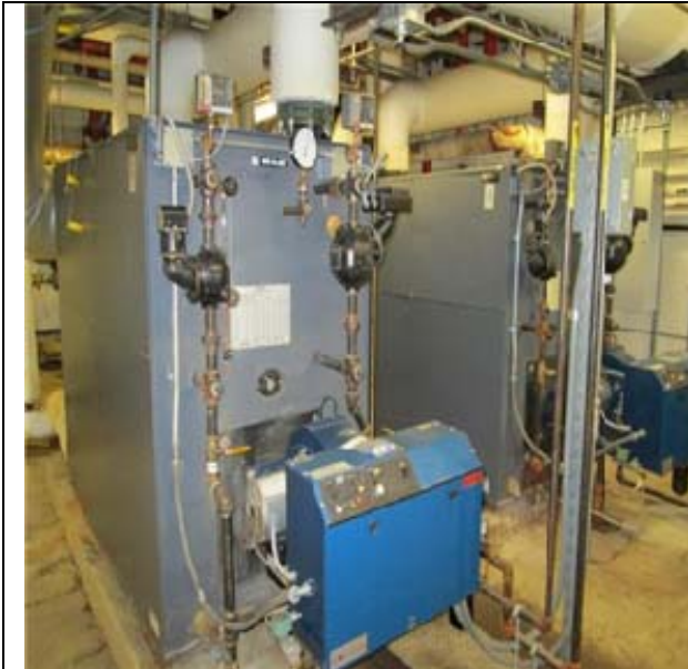
Oil-fired steam boiler, domestic hot water
