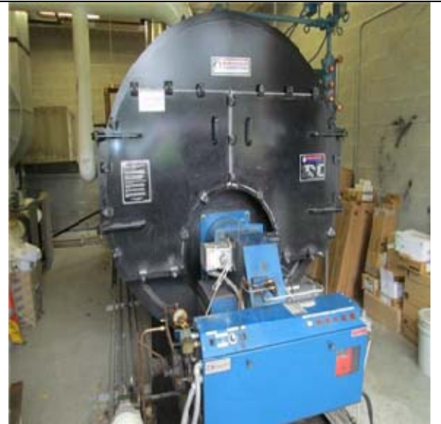
Oil-fired steam boiler
