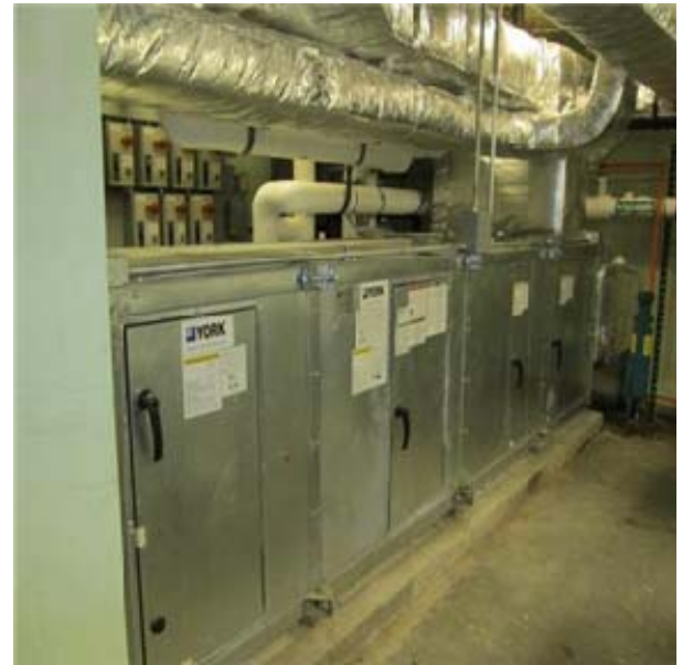
Common area AHU
