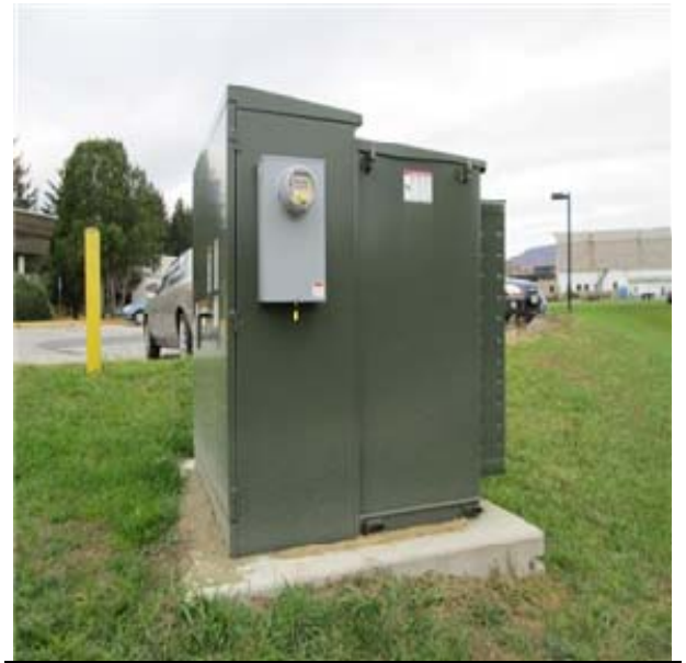
New service transformer
