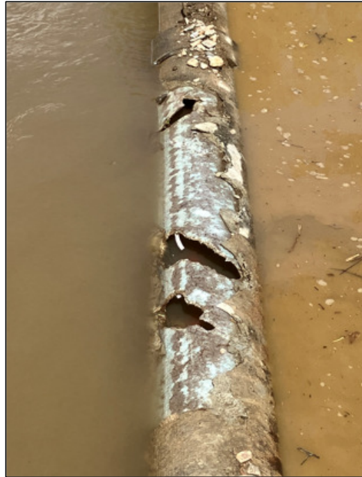
Broken 15" sewer line going into facility
