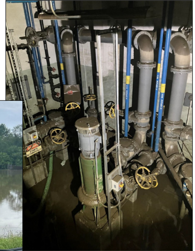
Influent pumps in basement
