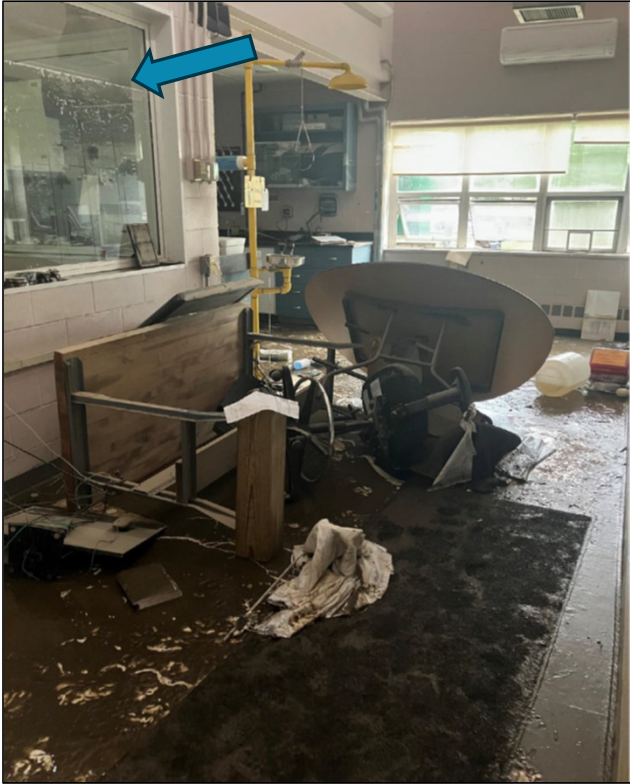
Control Room - Blue arrow points to high water mark
