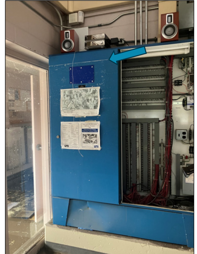
Programmable Logic Controller, white line at top is high water mark
