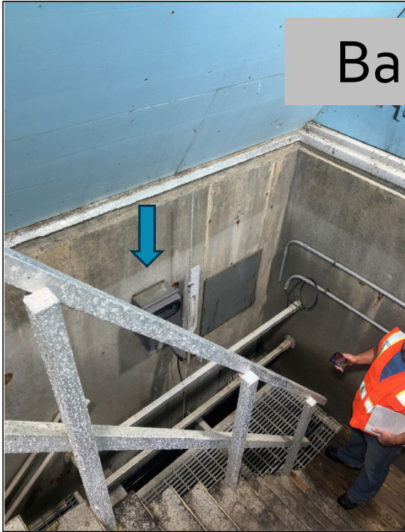
Lagoon overflowed into outfall building. Blue arrow shows high water mark above destroyed flow meter
