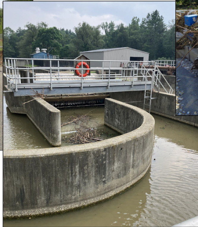
Flood Debris in Oxidation Ditch
