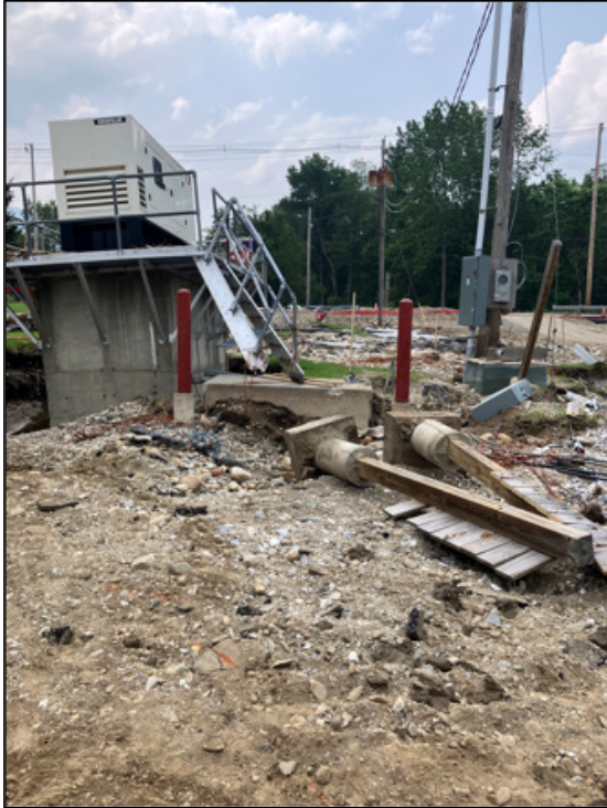
Generator built above current 500-year flood mark
