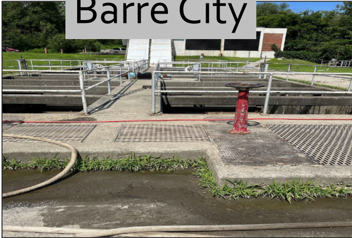
Primary Clarifiers – overflowed during flood
