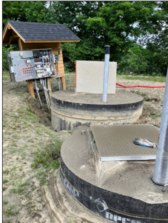
River Road West Pump Station completed in 2022 - water levels were over the control panel
