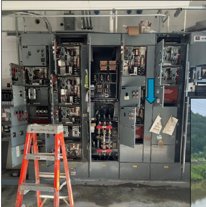
Motor Control Center – Blue arrow points to high water mark
