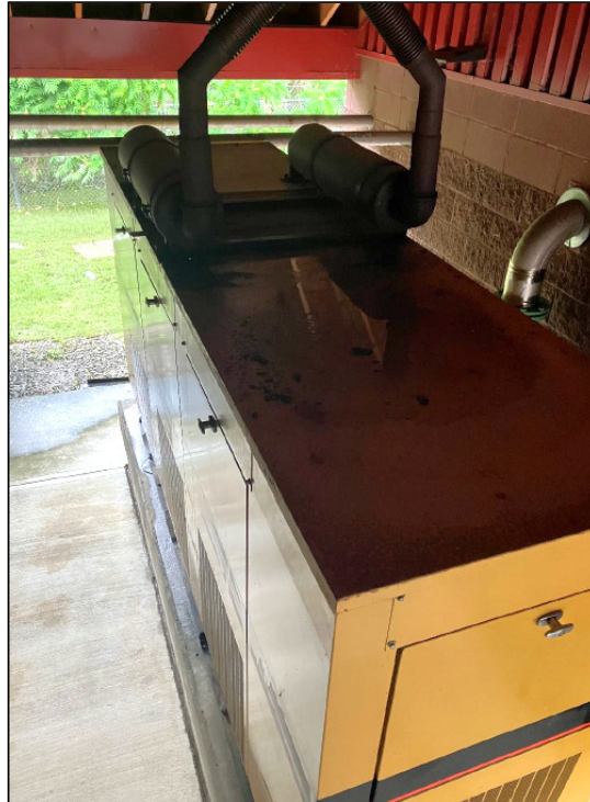
Generator - Remaining floodwater and silt on top
