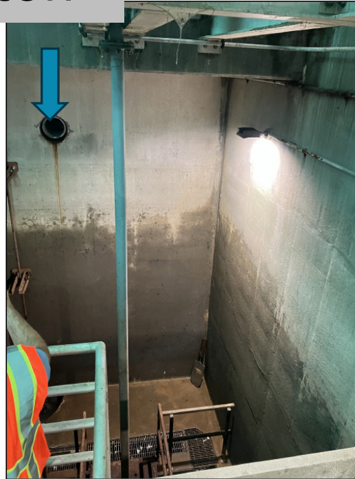
Main Pump Station – water levels rose to overflow pipe
