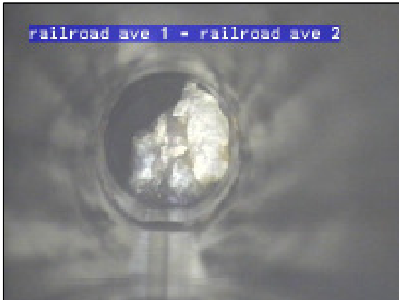
Johnson – blockage in pipe washed in from river during flood at line break
