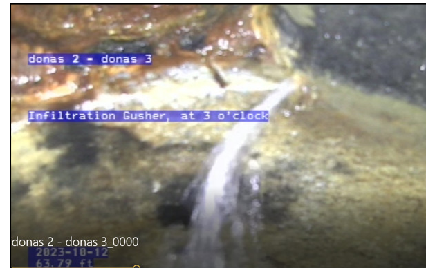
Hardwick – hole in pipe showing infiltration of groundwater
