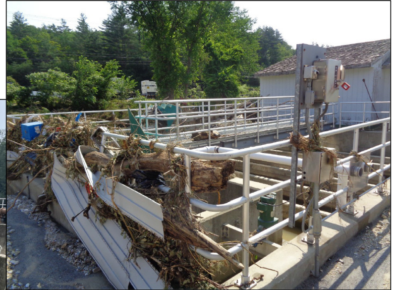
Flood Debris at Chlorine Disinfection Contact Chamber
