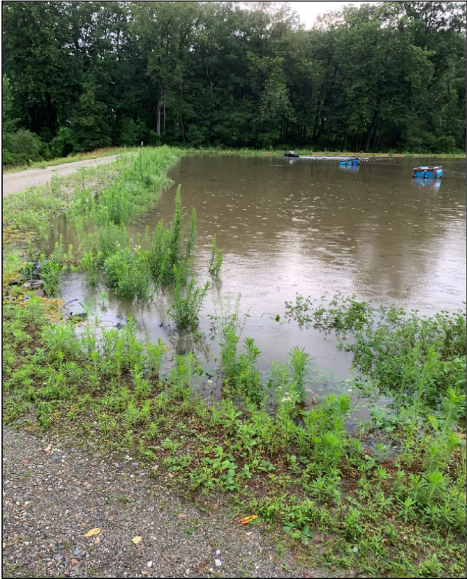
Lagoon 1 beginning to flood
