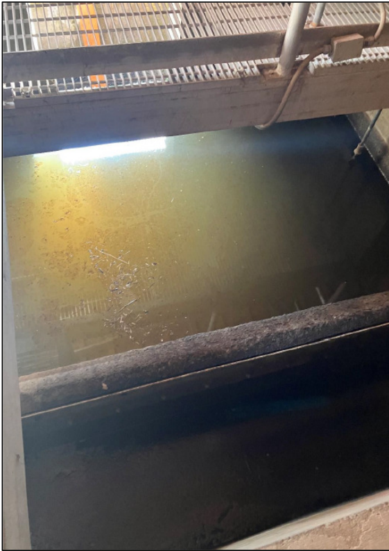
Floodwater in Ultraviolet Disinfection Chamber
