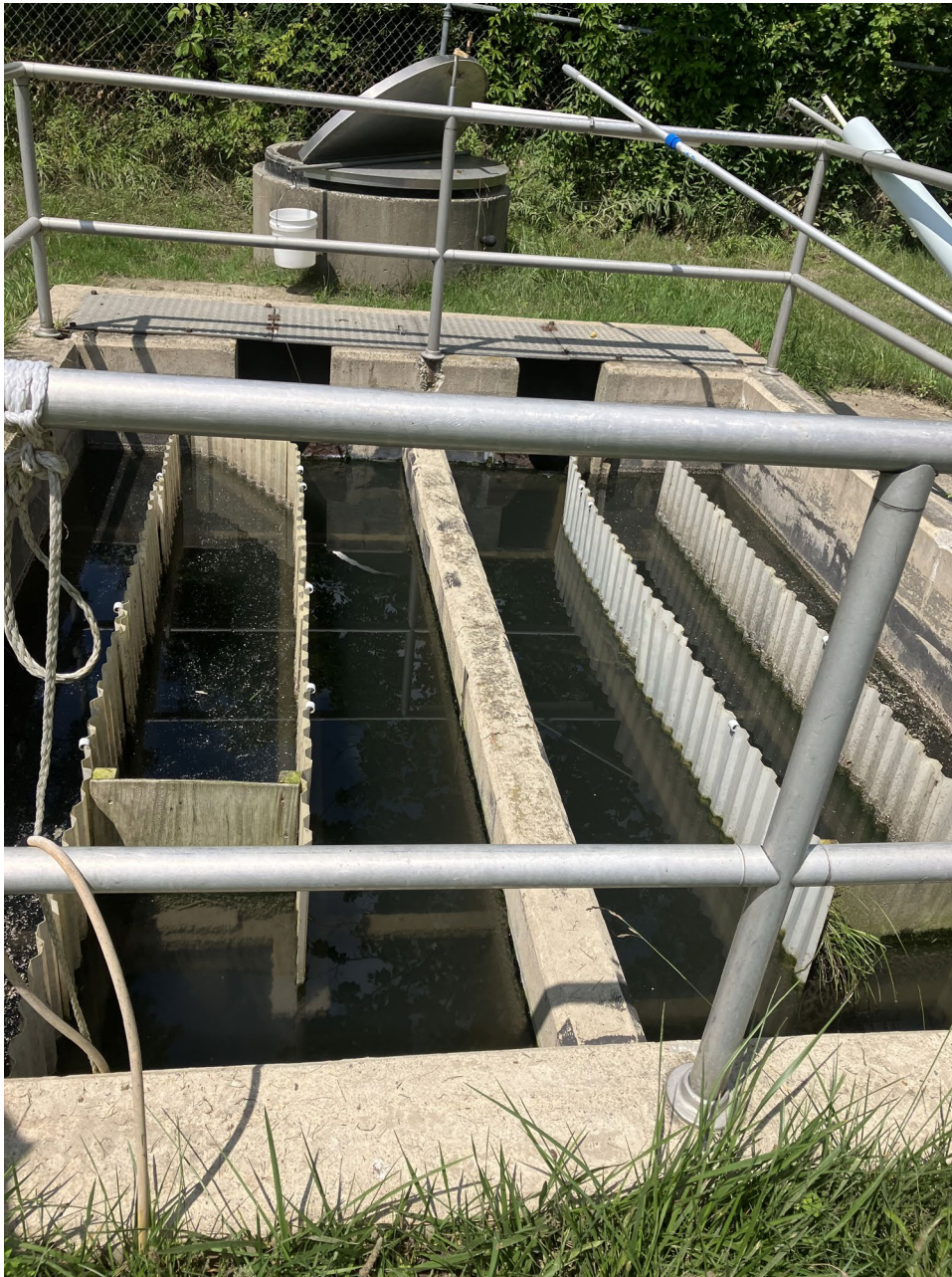
6-Chlorine Contact Chamber
