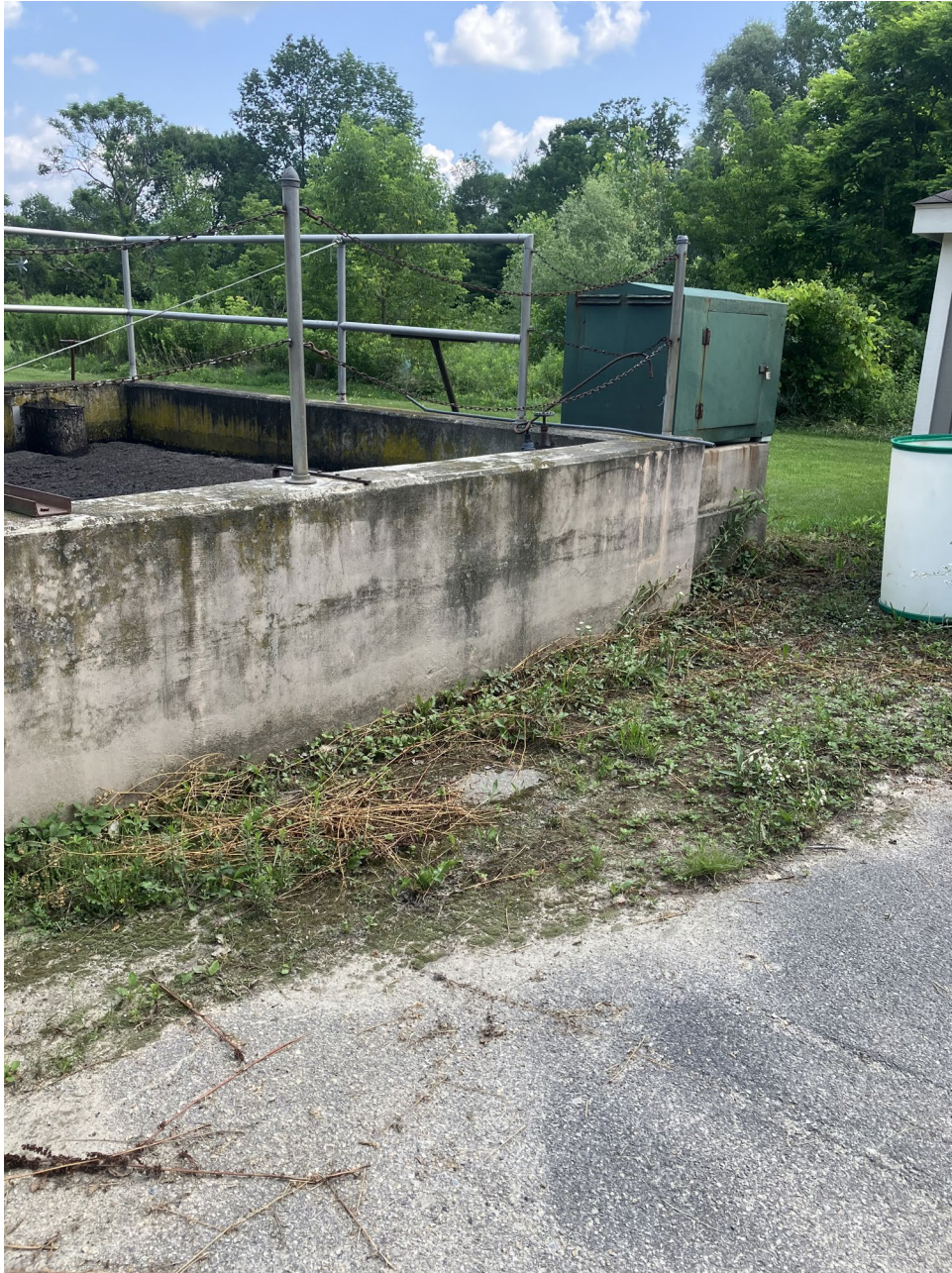
9- Aerated Sludge Holding Tank with High Water Mark Line Approximately 2 feet
