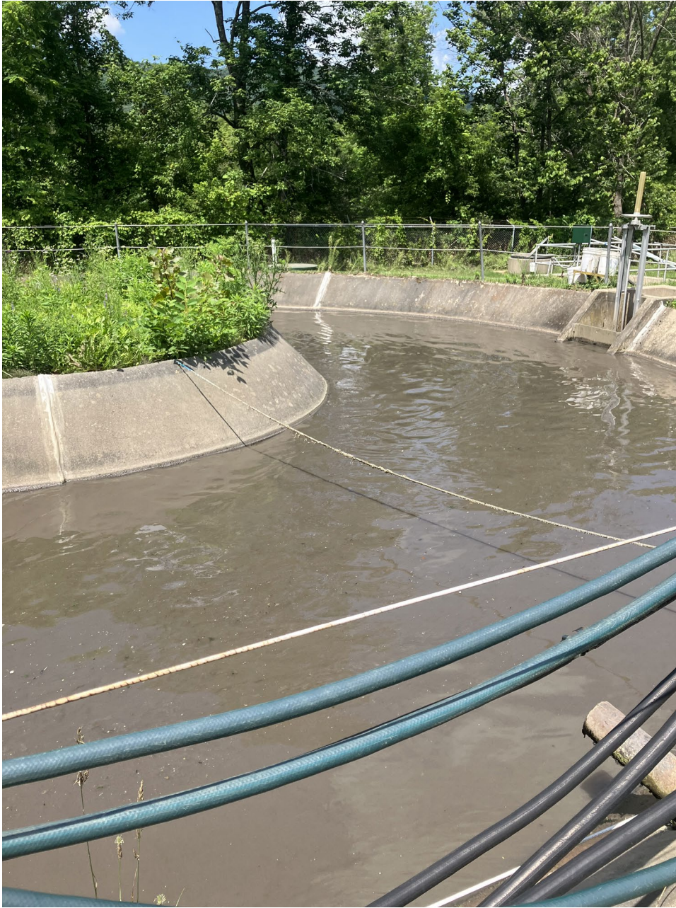
3-Oxidation Ditch with Residual Debris
