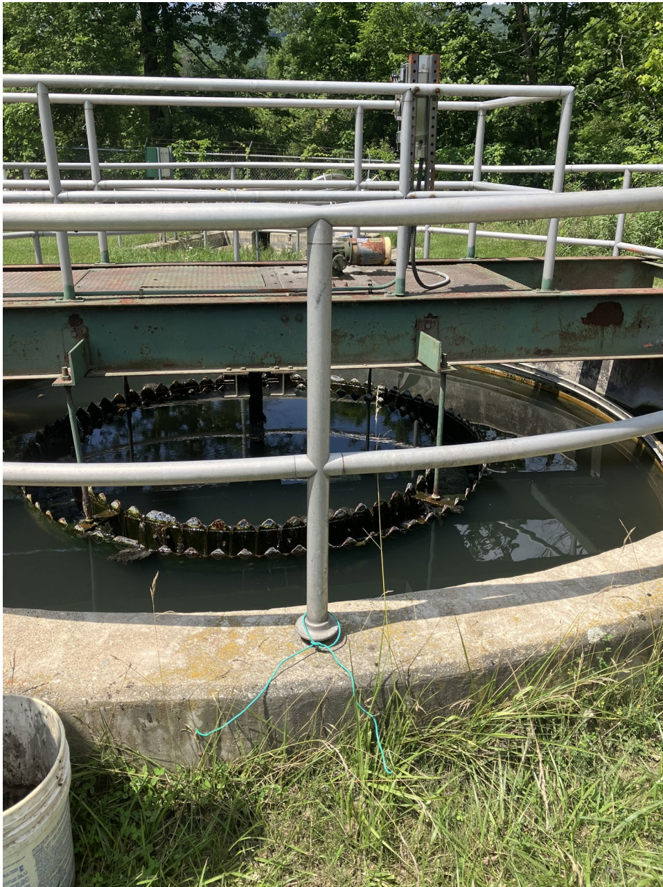
5-Clarifier Converted to Contact Chamber
