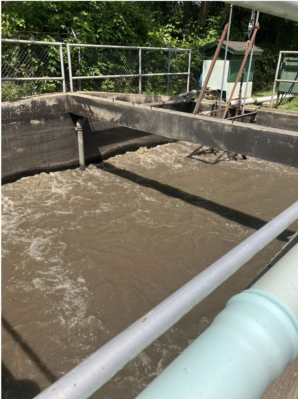
8- Aerated Sludge Holding Tank
