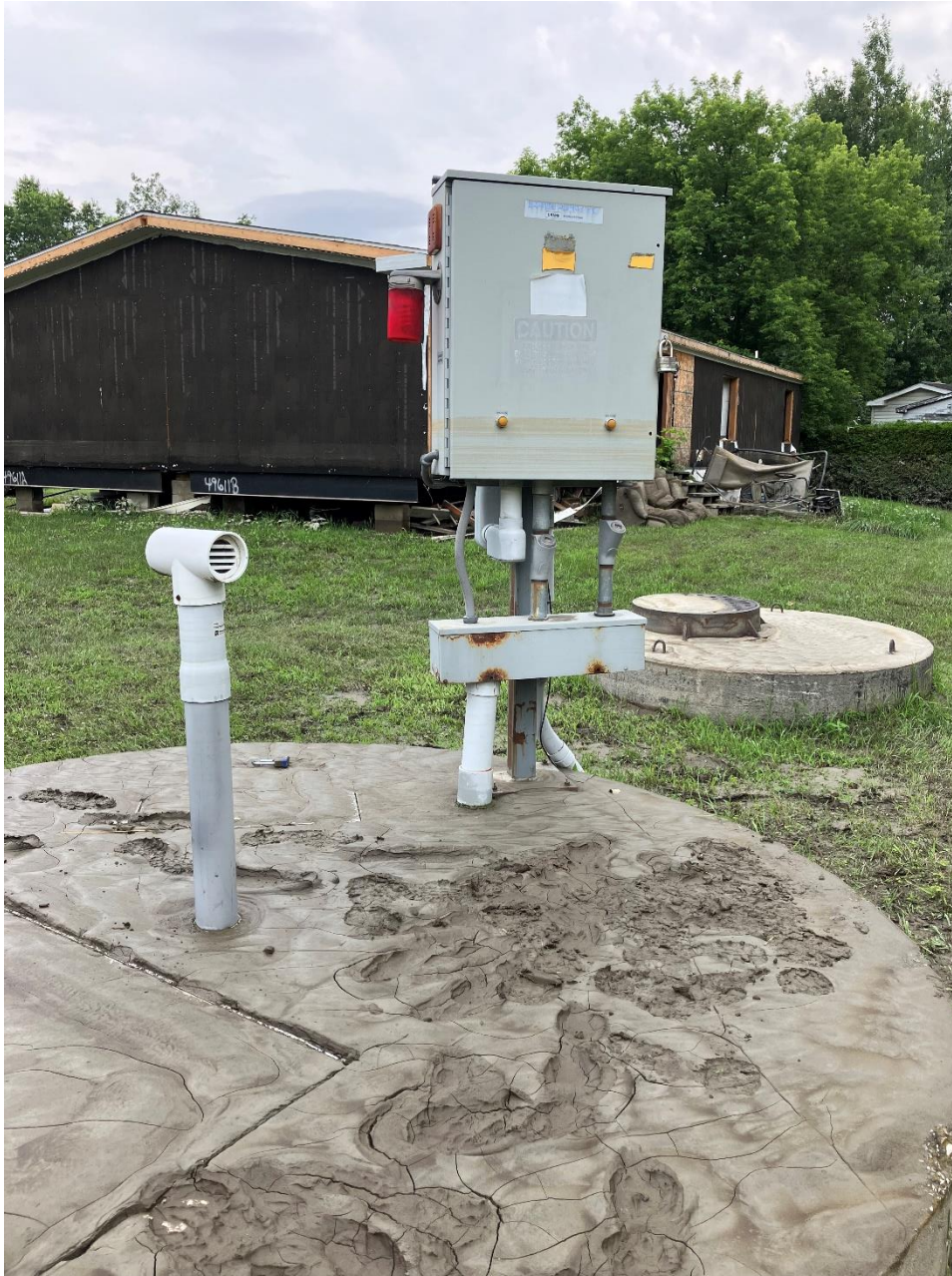
26- Highland Heights Pump Station
