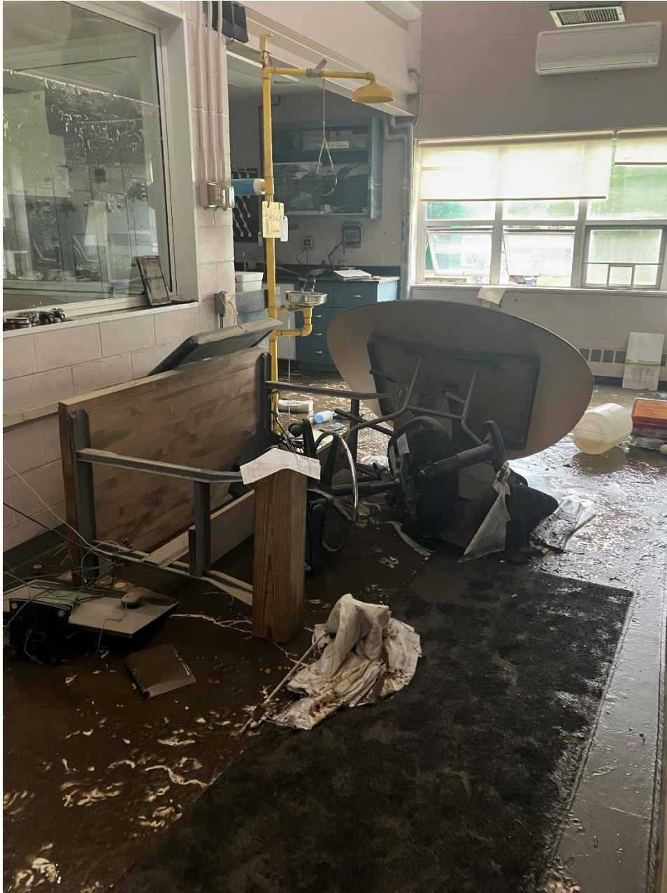
3- Post Flood Debris in Control Room
