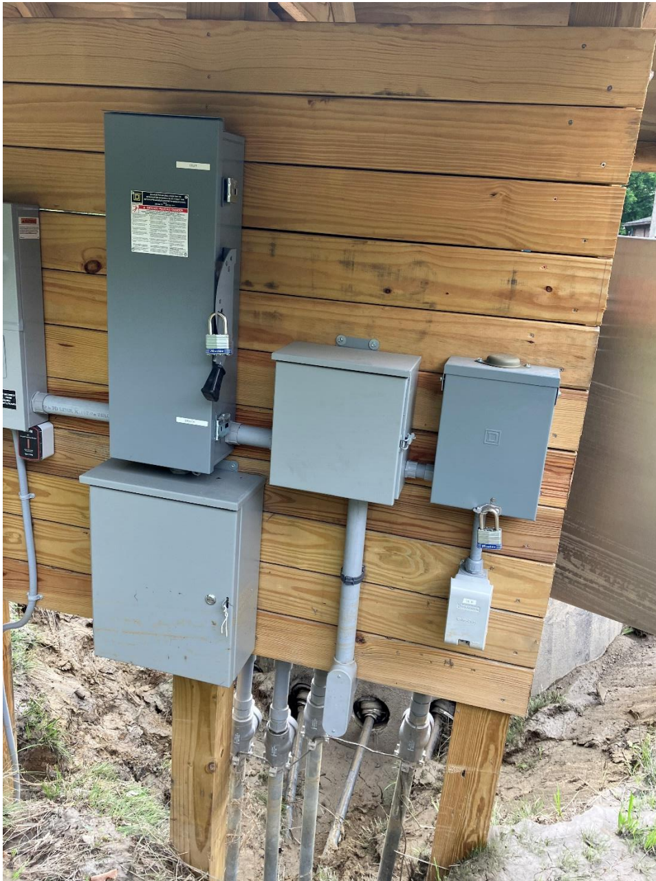
24- River Road West Pump Station Back of Electrical/Control Panel Mount
