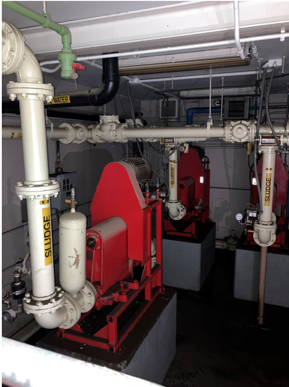
16- Sludge Pump Room
