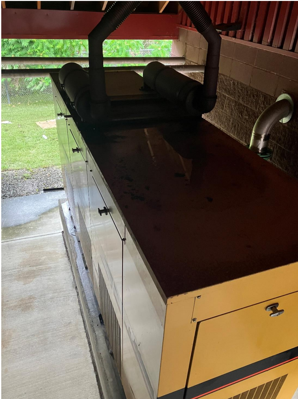
14- Plant Generator Top View Showing Residual Floodwater and Silt on Top
