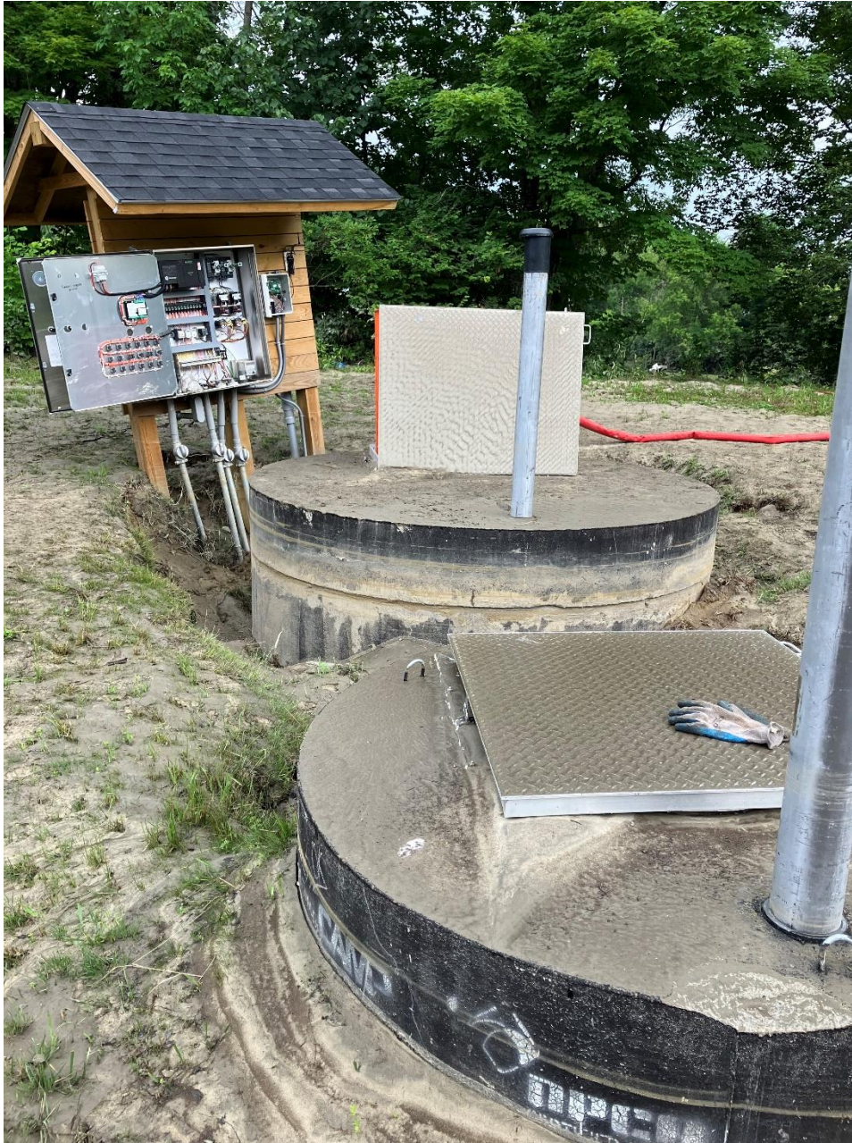
23- River Road West Pump Station
