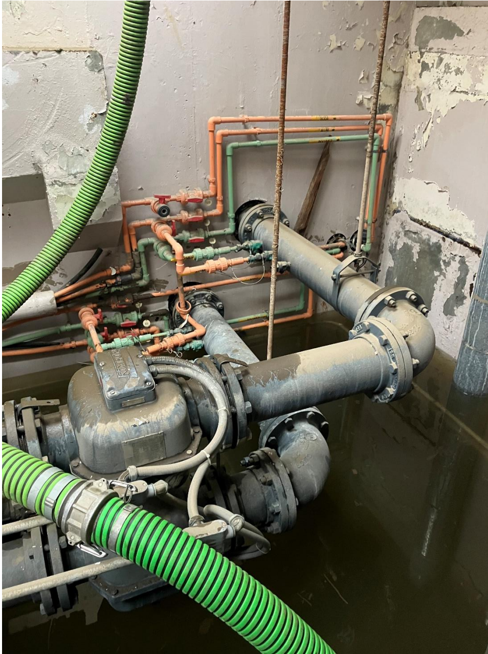
17-Influent Dry Well Piping with Influent Pumps Below Water Level
