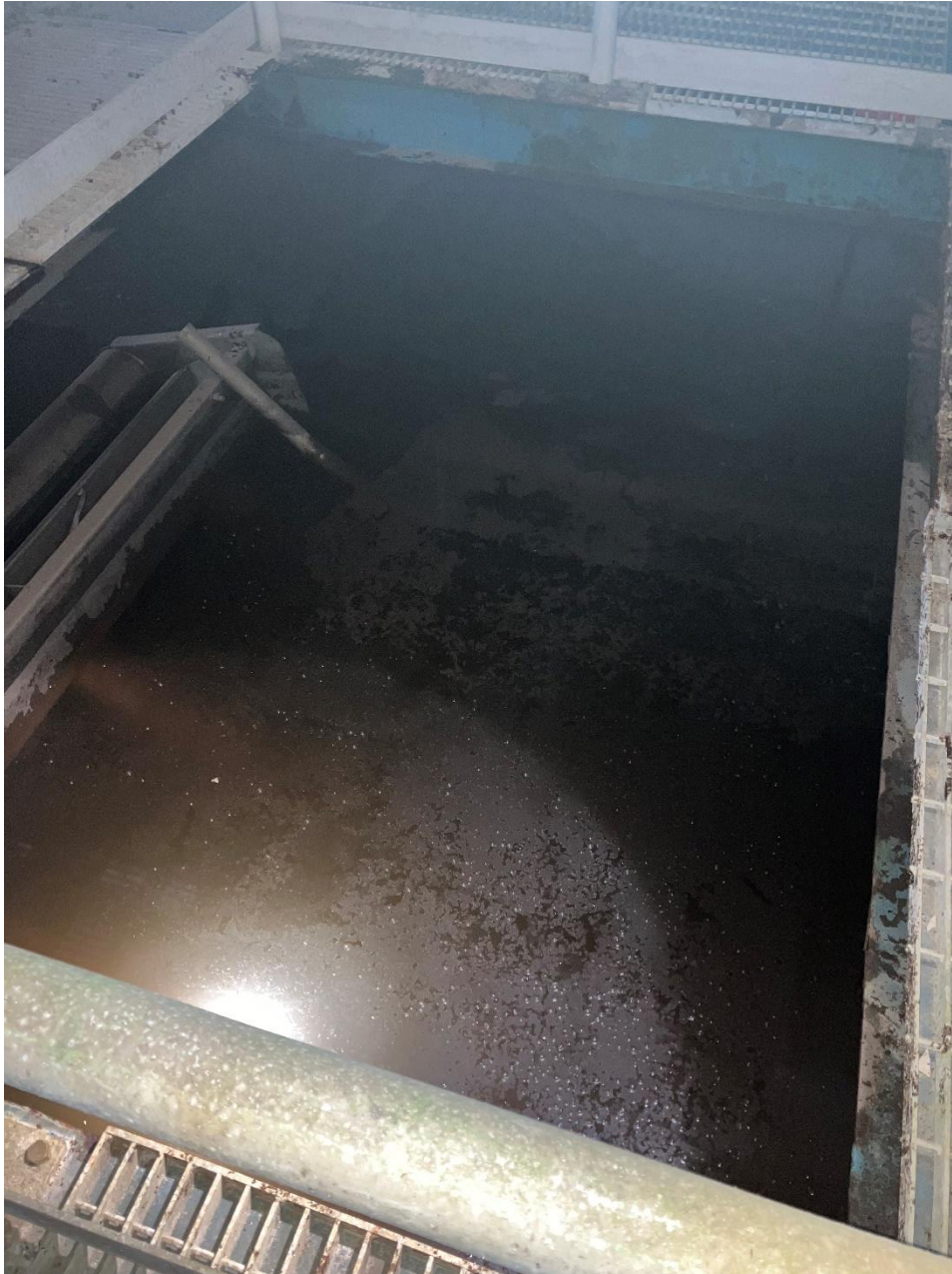
18- Sequencing Batch Reactor (SBR) Chamber with Decanter
