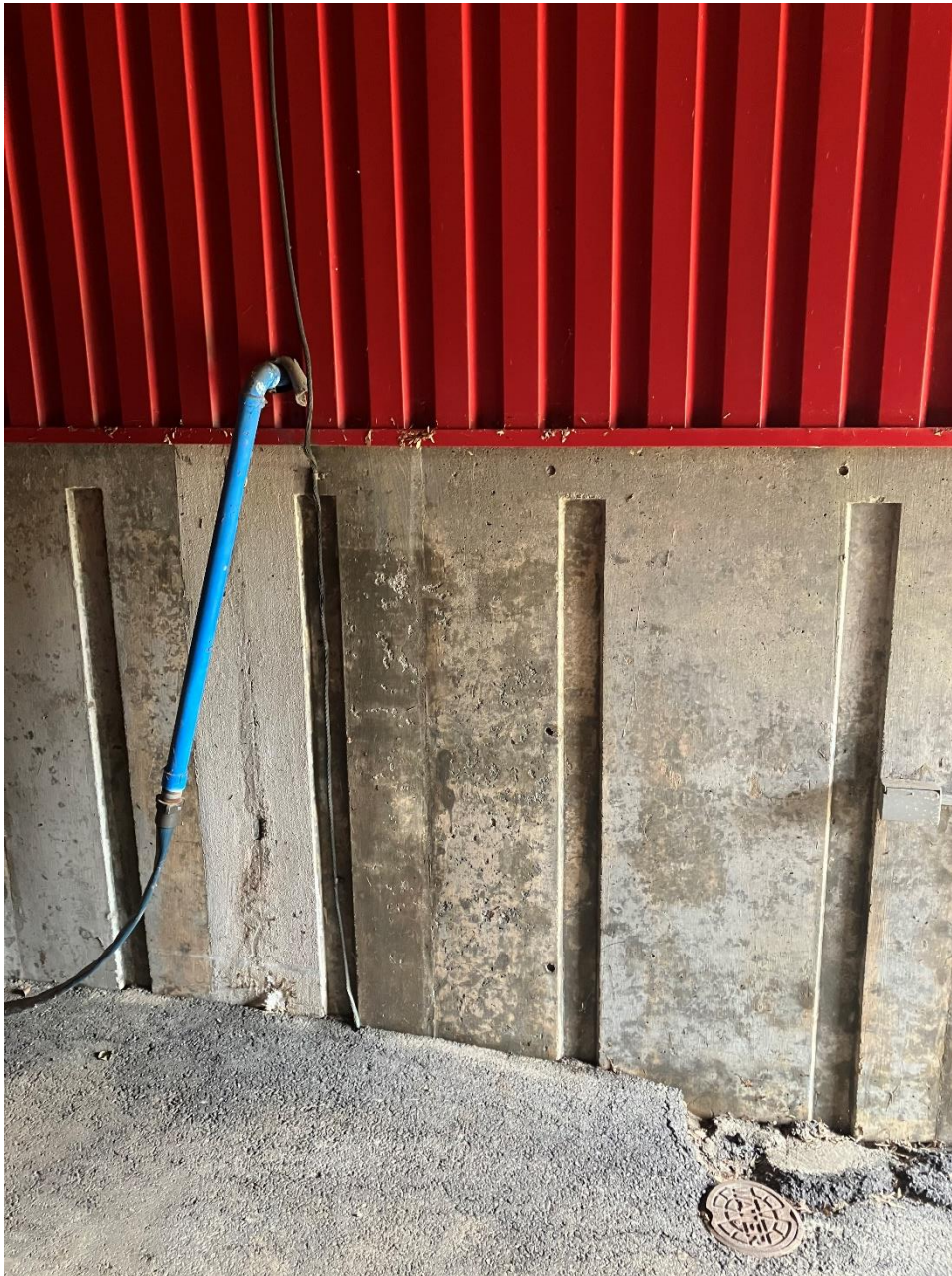
21- UV Building High Water Mark (Almost Even with Blue Pipe)
