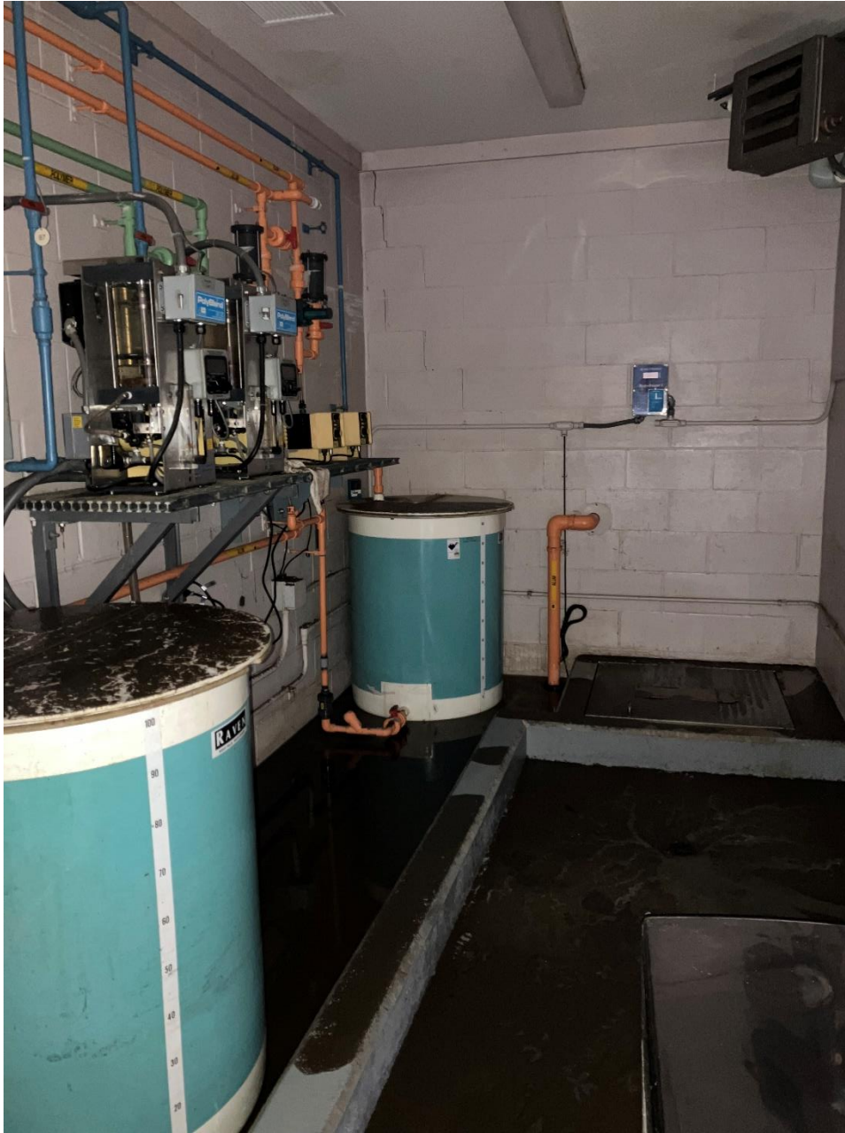
11- Chemical Feed Room with Tanks and Pumps
