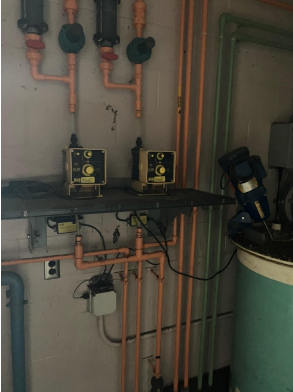
12- Chemical Feed Room with Additional Pumps and Feed Lines
