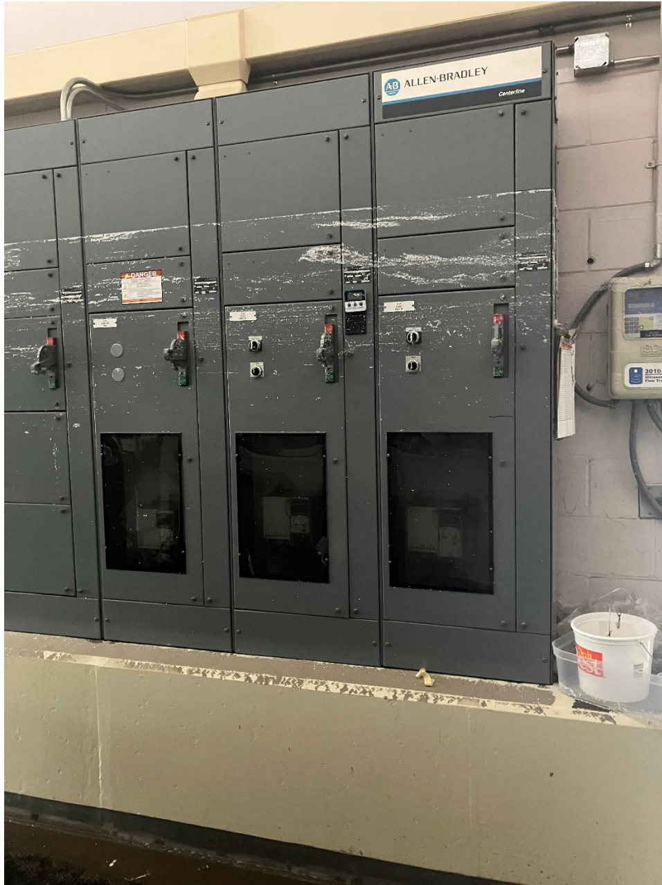
1 - High Water Mark on MCC
