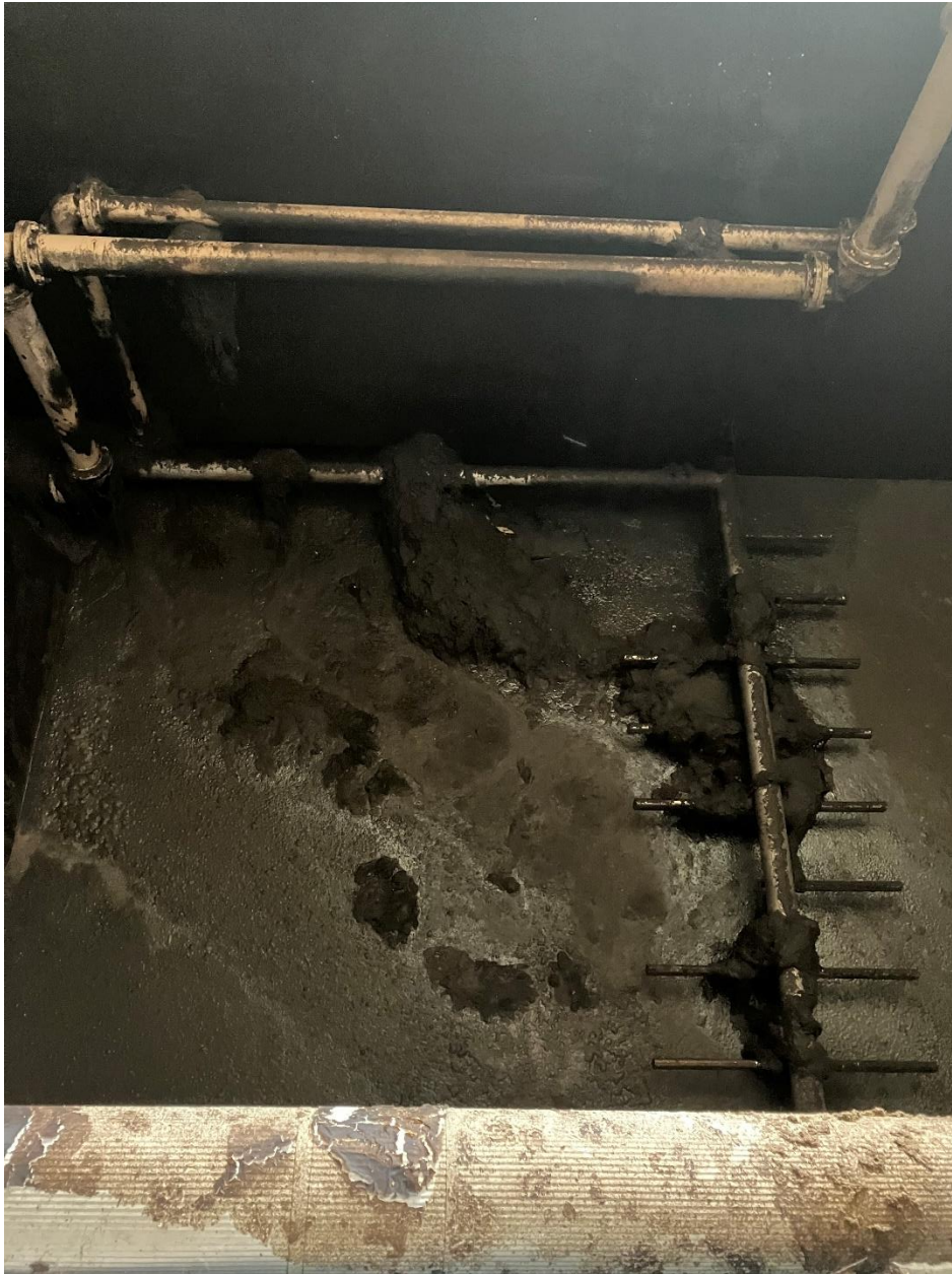
19- SBR Chamber After Pumping Out Flood Waters
