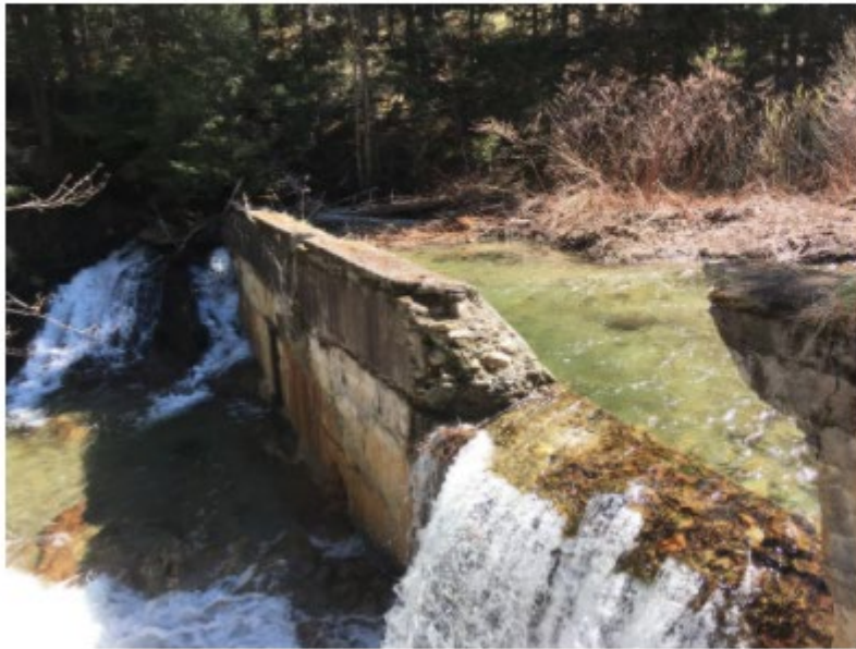
Before removal of Camp Wihakowi dam on Bull Run river in Northfield, VT.
