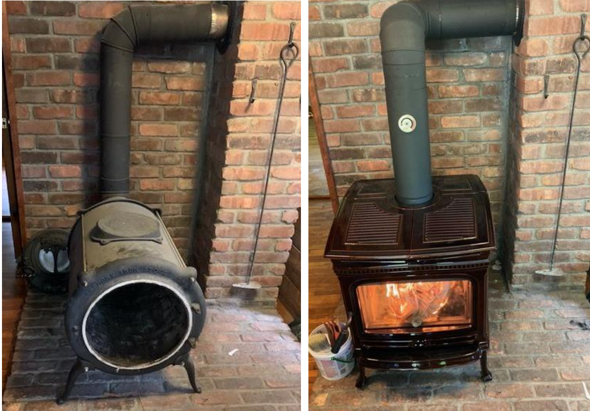
Figure 8. Photos of an old cord wood stove (left) removed, and a new cord wood stove installed (right)
