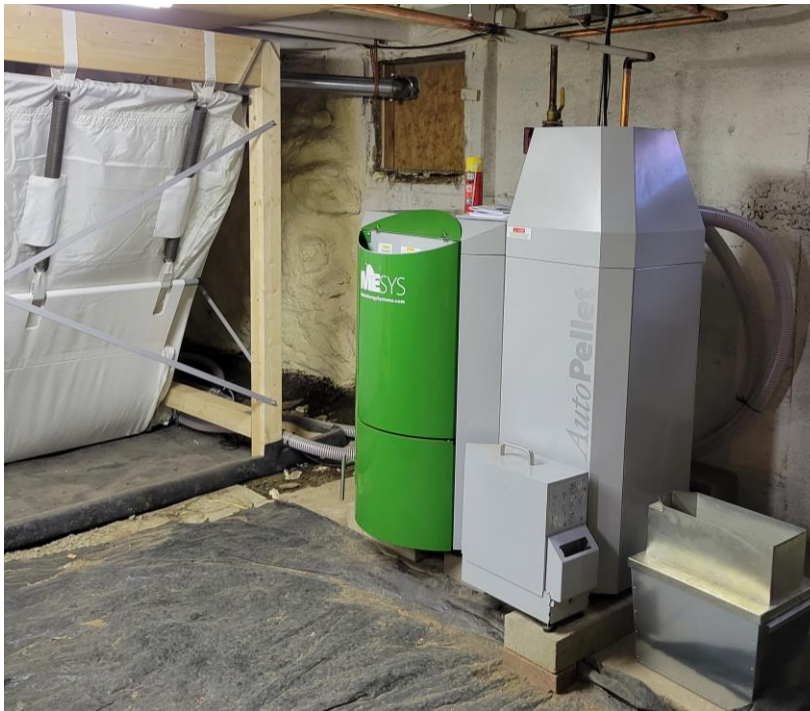
Figure 6. Photo of old coal boiler (above) and new pellet boiler and pellet storage bag (below)
