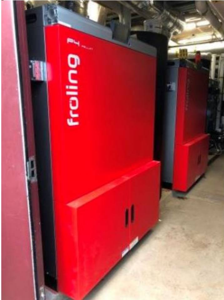
Figure 9. New Froling pellet boilers at the Dummerston School
