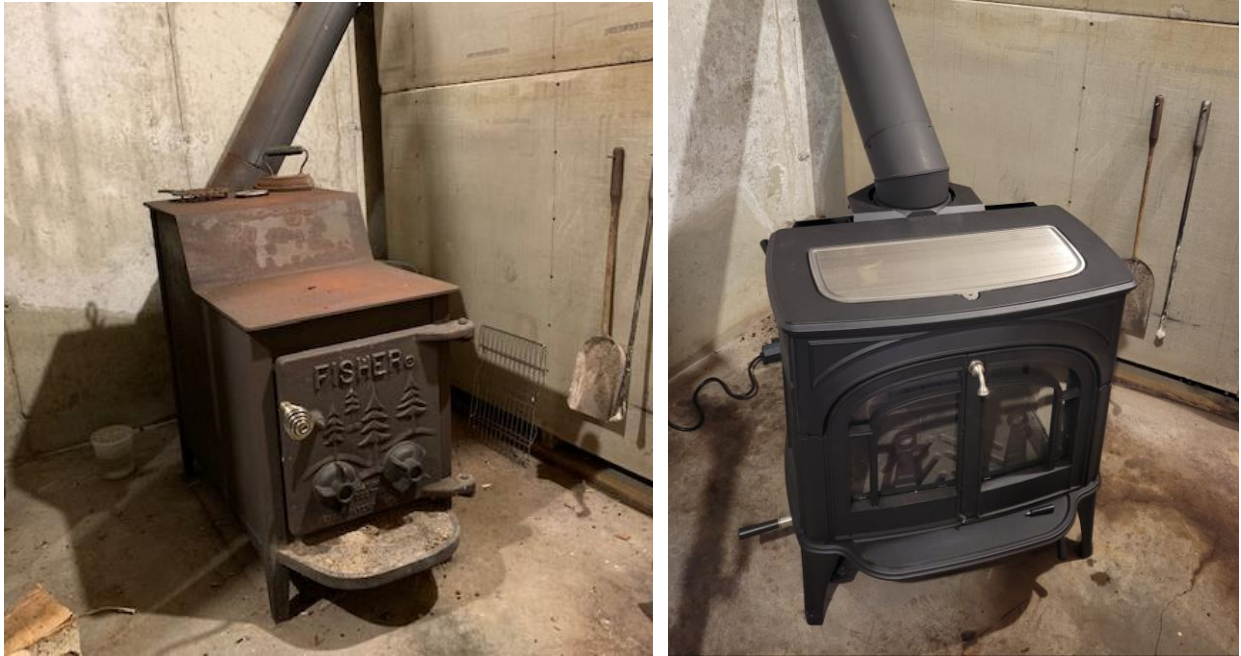
Figure 7. Photos of an old cord wood stove (left) removed, and a new pellet stove installed (right)
