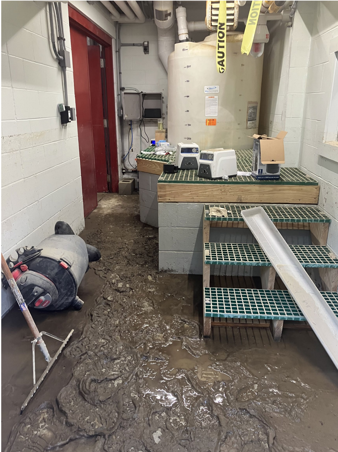
26- Main Control Building Chlorine Tank. Note High Water Mark at Approximately 4 feet.
