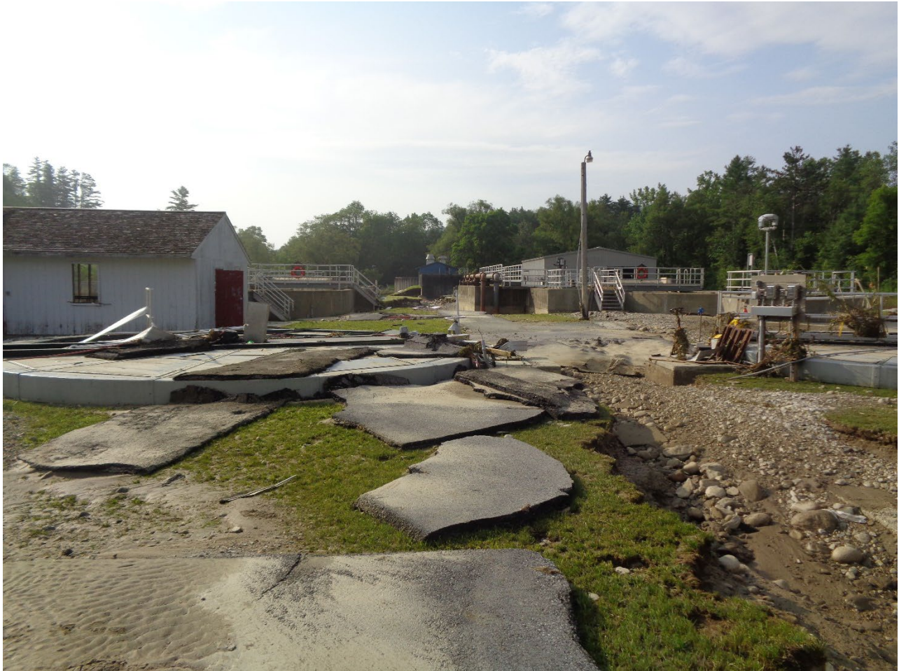
11 – Left Side: Clarifier No. 1 With Displaced Asphalt Around and on Top of Clarifier. Right Side: Clarifier No. 2. Looking Towards Oxidation Ditches. Note Extreme Scour (Photo courtesy of Aldrich and Elliot, PC)
