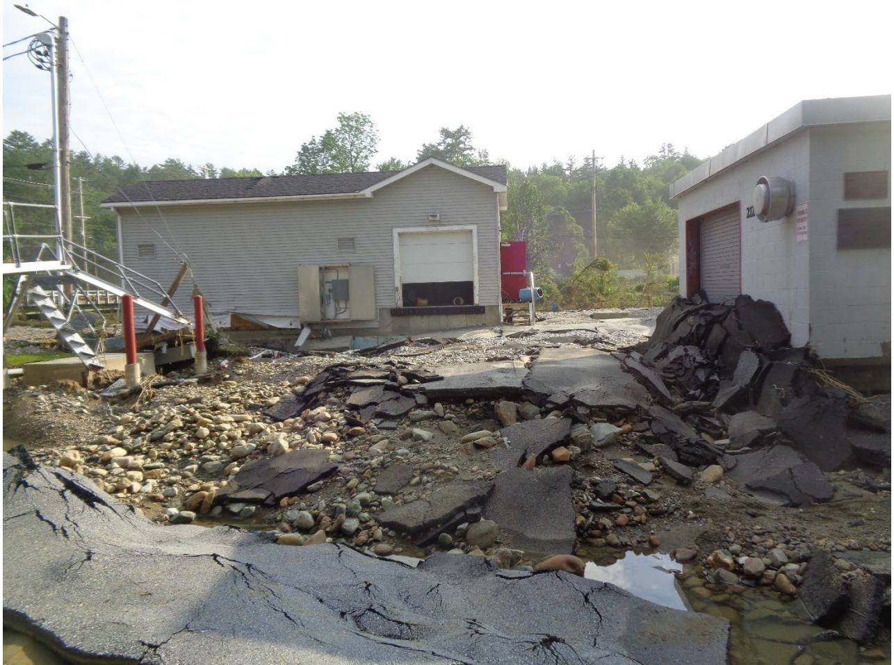
3 – Left Side: Headworks Building, Right Side Main Control Building. Displaced Asphalt Deposited and Extreme Scour (Photo courtesy of Aldrich and Elliot, PC)
