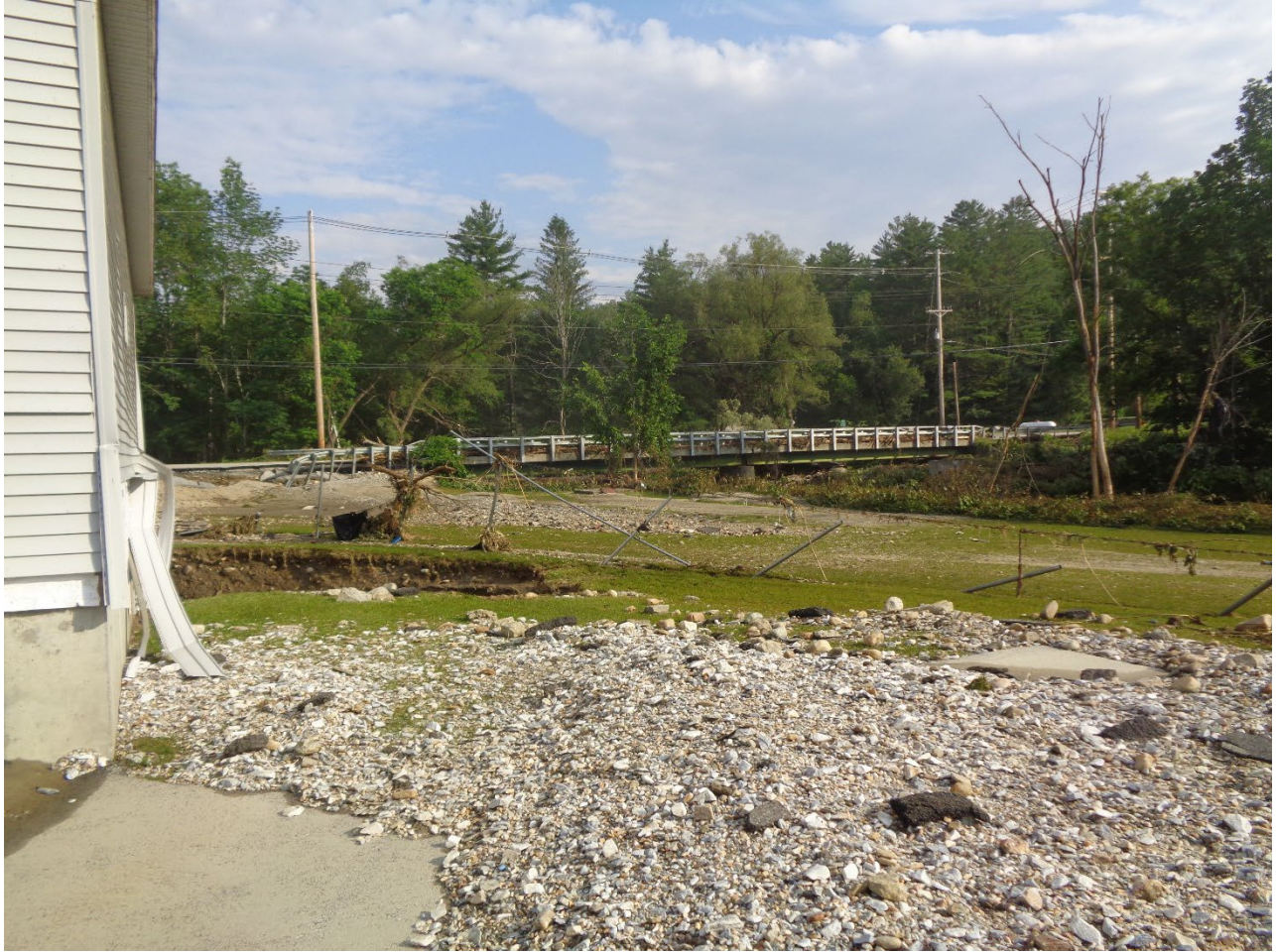
4 – Left Side: Headworks Building, Looking Back Towards Entrance. Extreme Scour and Site Fence Damage (Photo courtesy of Aldrich and Elliot, PC)
