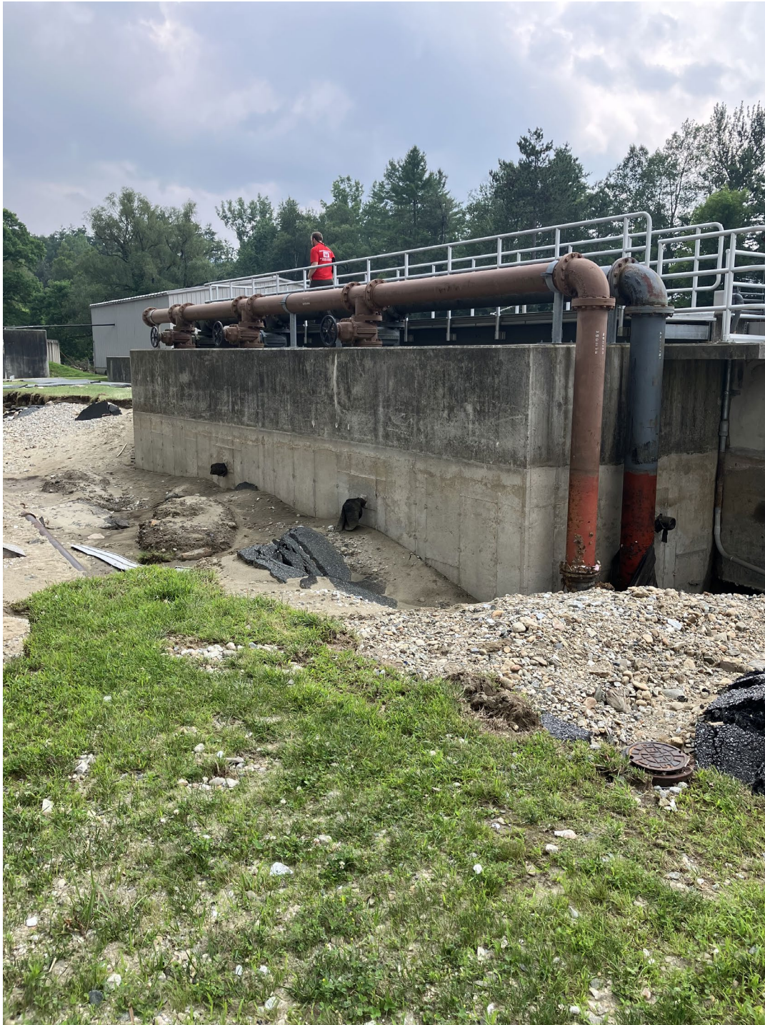
16 –West Oxidation Ditch Exterior. Note Extreme Scour
