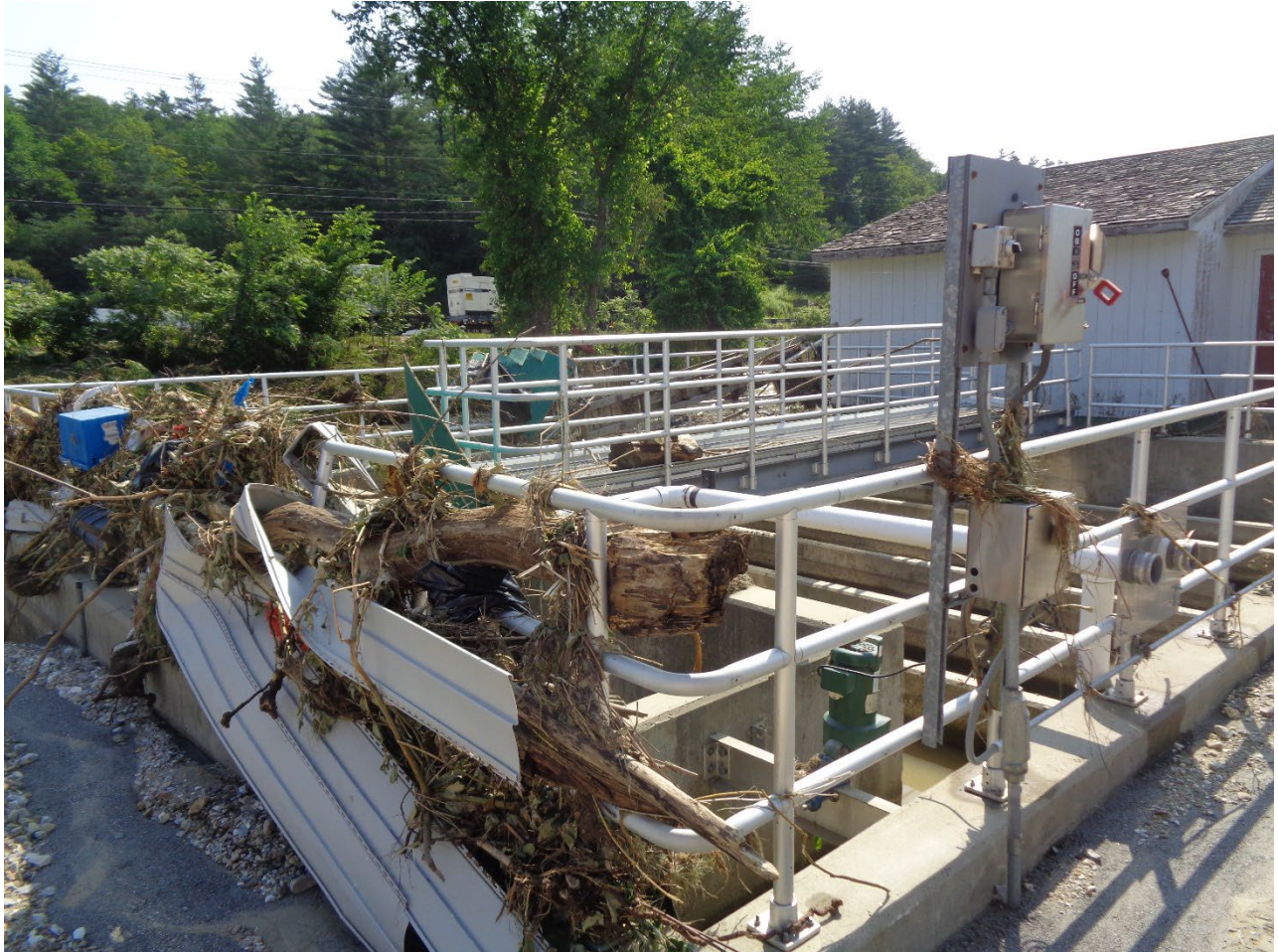
20 –Chlorine Contact Chamber. Note Extreme Scour and Debris (Photo courtesy of Aldrich and Elliot, PC)
