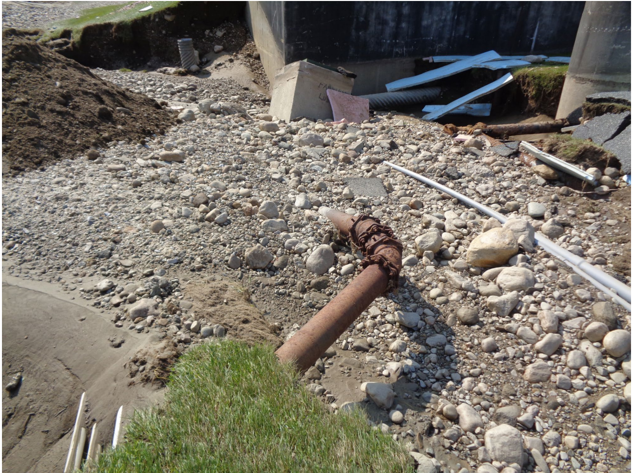
24- Aerobic Digester. Note Exposed Piping and Conduits (Photo courtesy of Aldrich and Elliot, PC)
