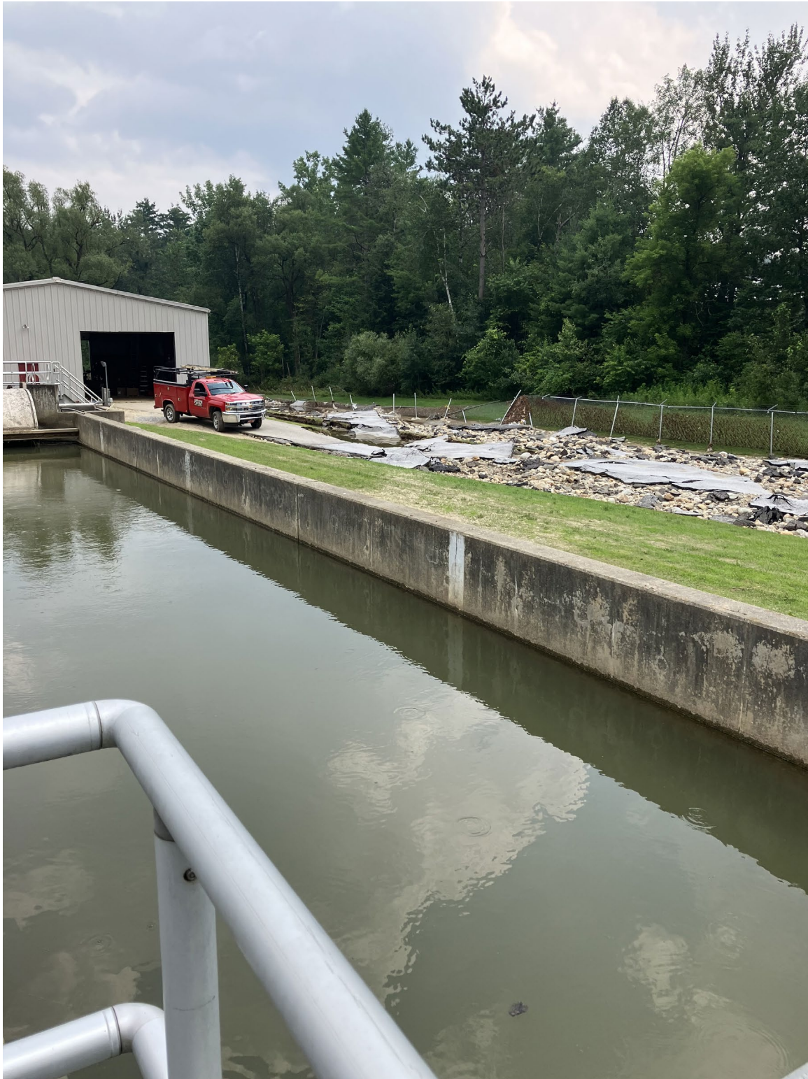
19 –West Oxidation Ditch Interior. Note Extreme Scour Along Drive and Damaged Fencing Behind Oxidation Ditch
