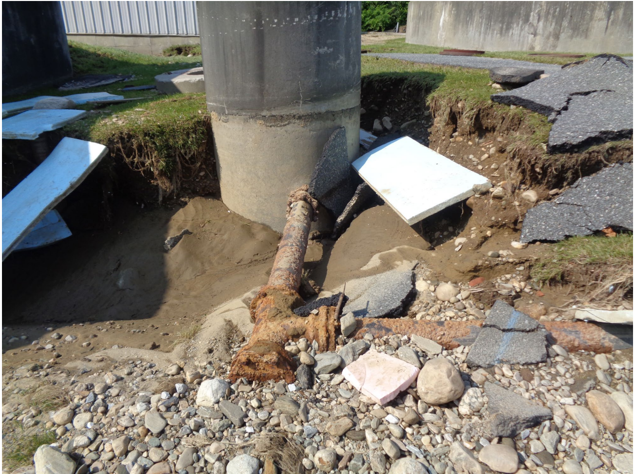
25- Aerobic Digester. Note Exposed Piping Scour and Debris (Photo courtesy of Aldrich and Elliot, PC)
