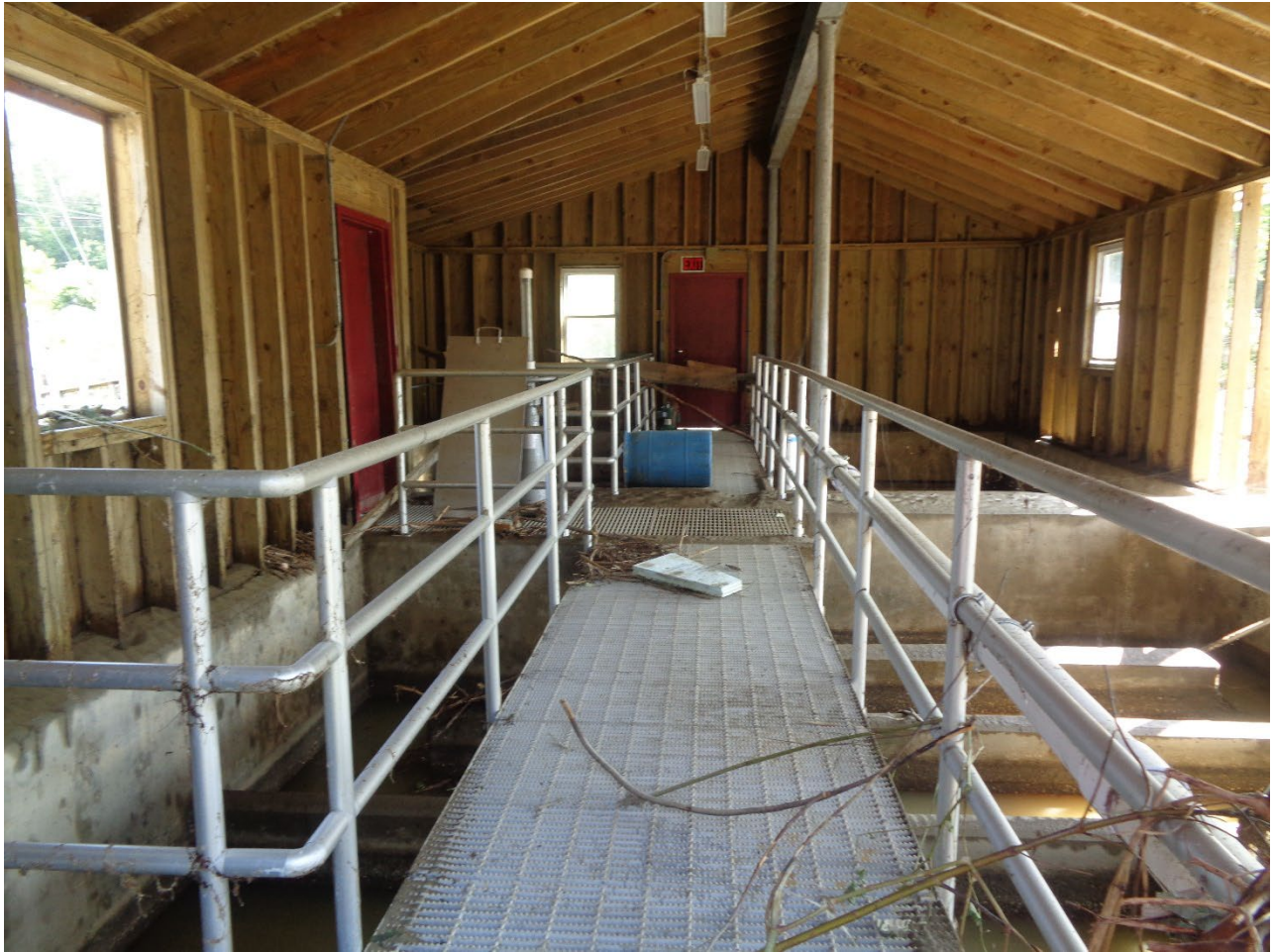
22 –Chlorine Contact Tank Building Interior. Note Window Missing on Left Side and Debris
