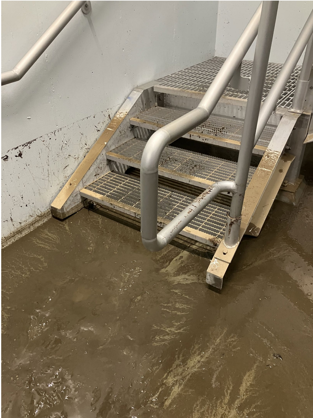
9 – Basement Area of Influent Pump Station Showing High Water Mark at Approximately 18”.
