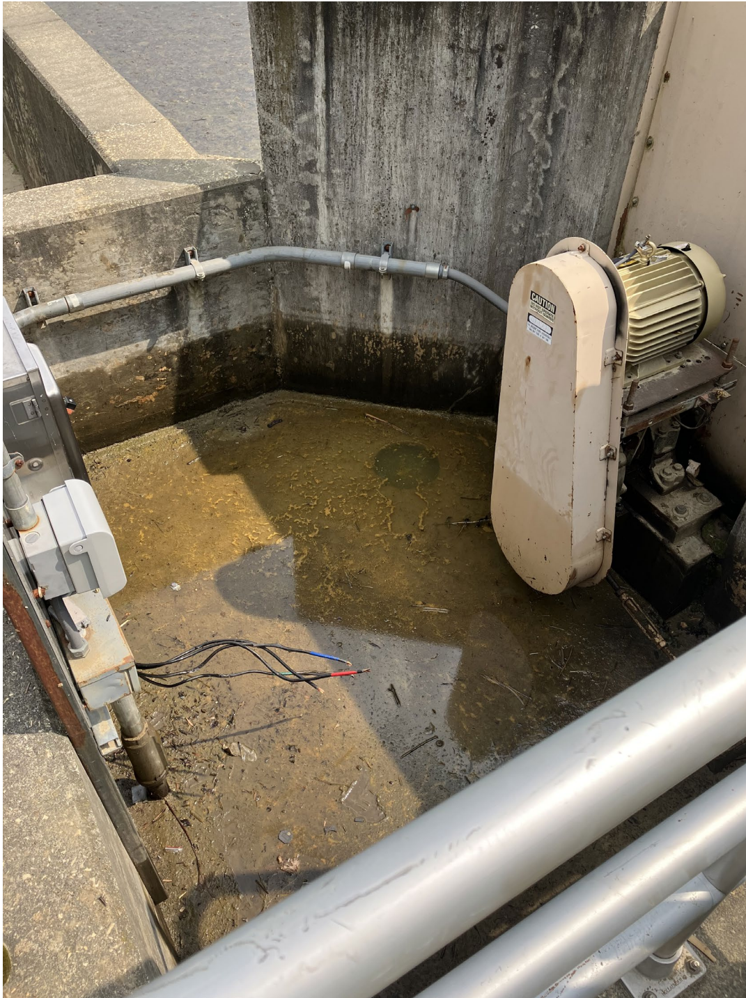
18 –Rotary Drum Motor in West Oxidation Ditch Interior. Note Debris
