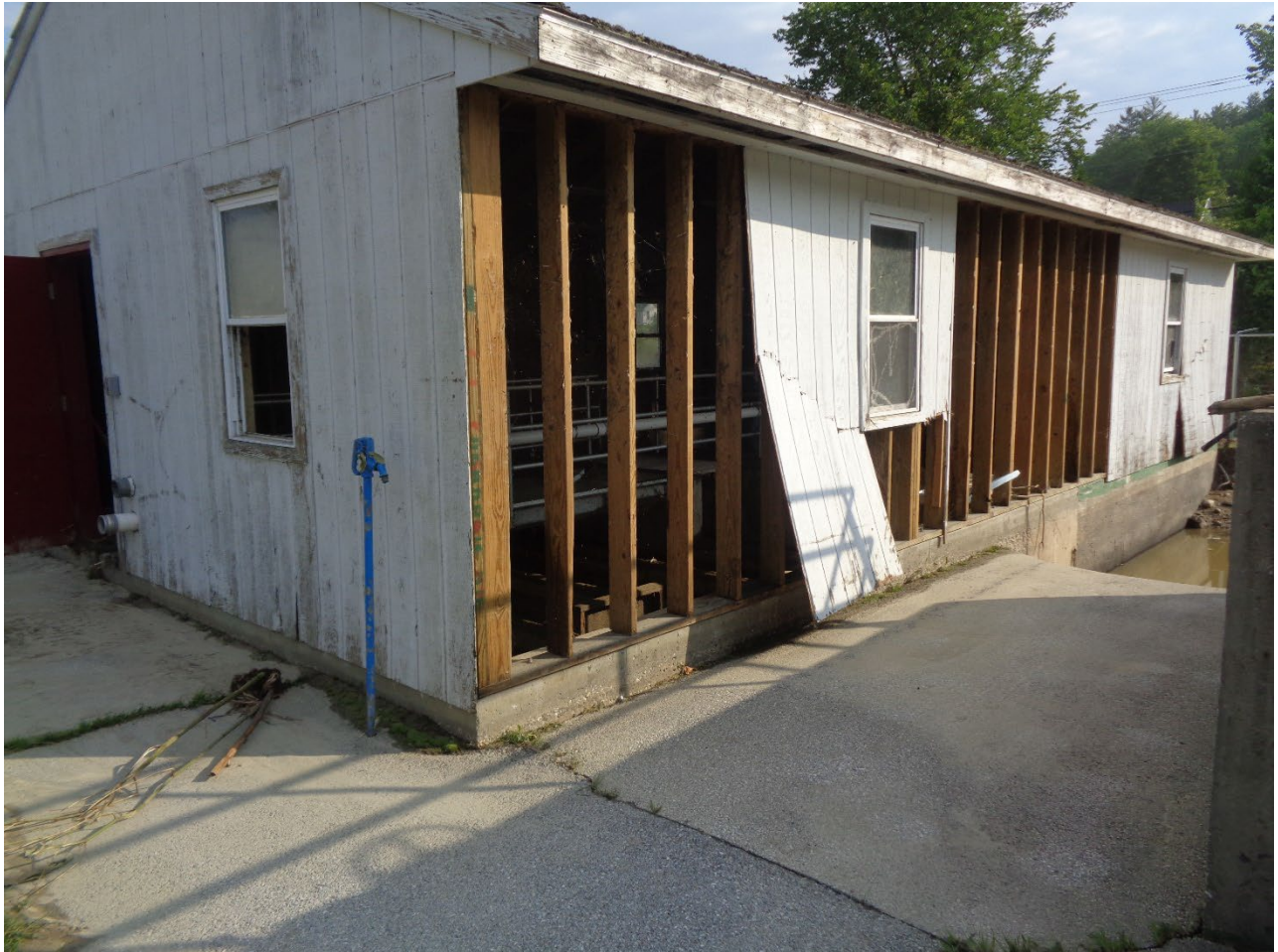
21 –Chlorine Contact Tank Building. (Photo courtesy of Aldrich and Elliot, PC)
