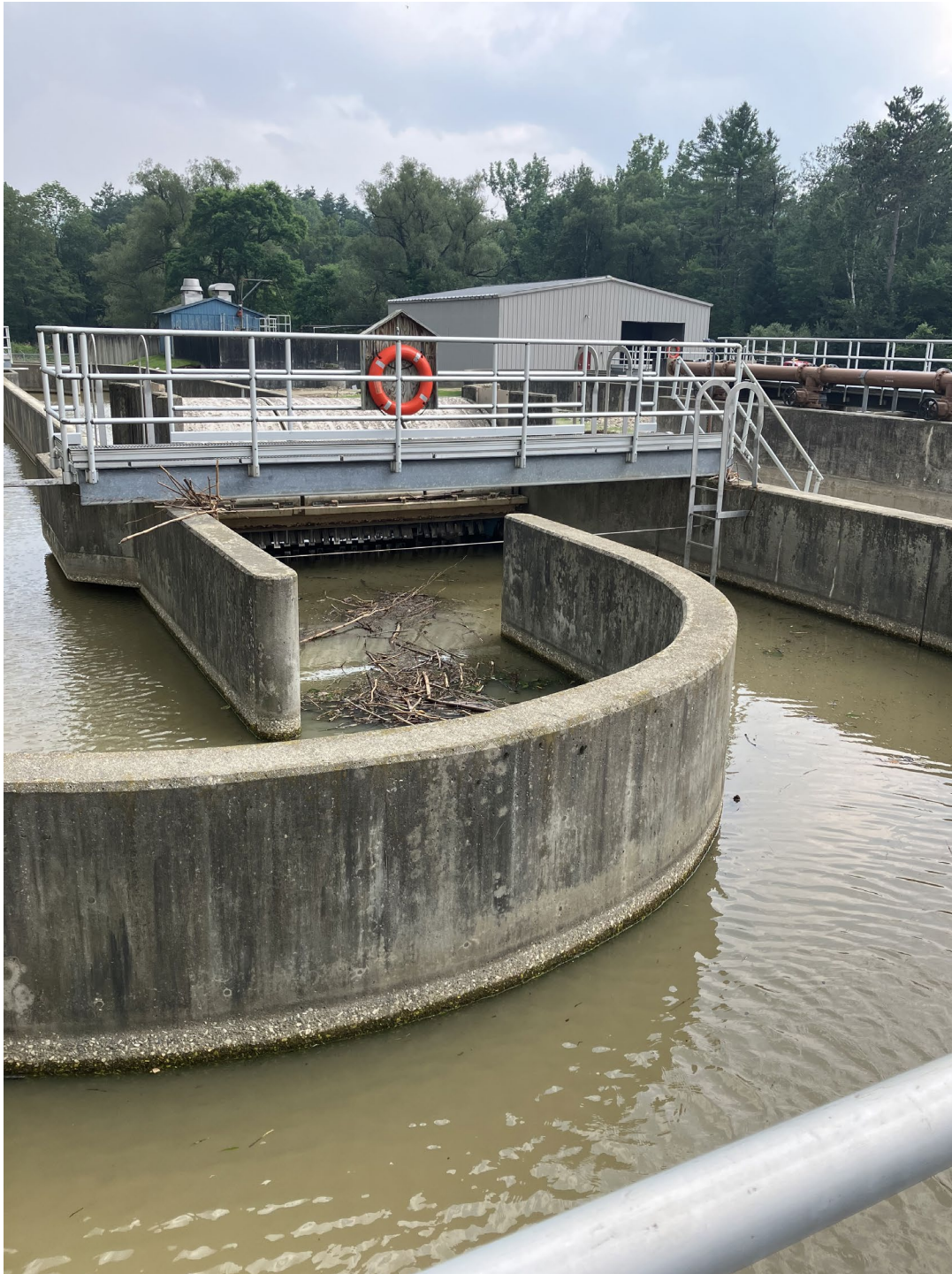
15 –East Oxidation Ditch Interior. Note Debris
