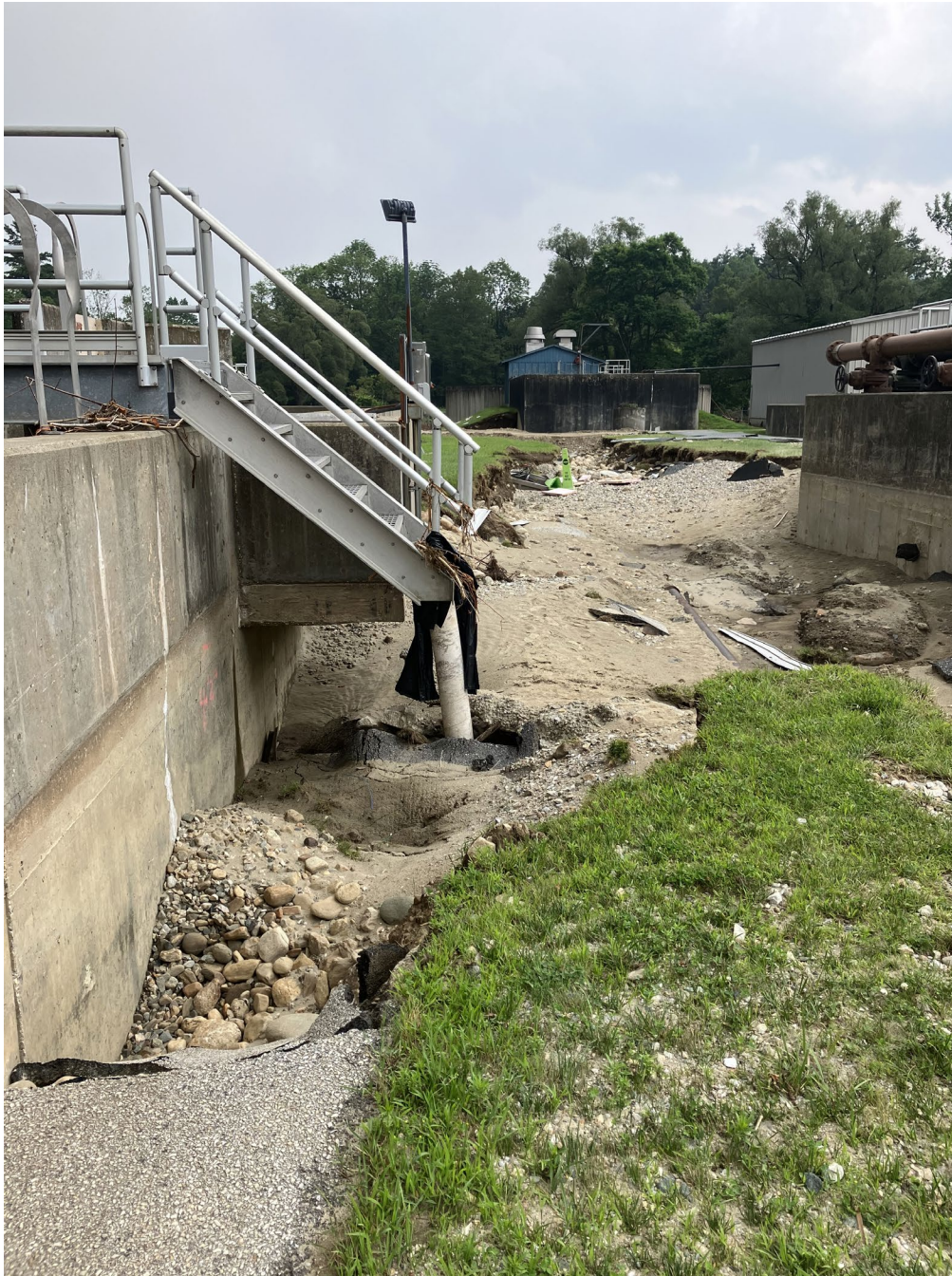
14 –East Oxidation Ditch Exterior. Note Debris and Extreme Scour
