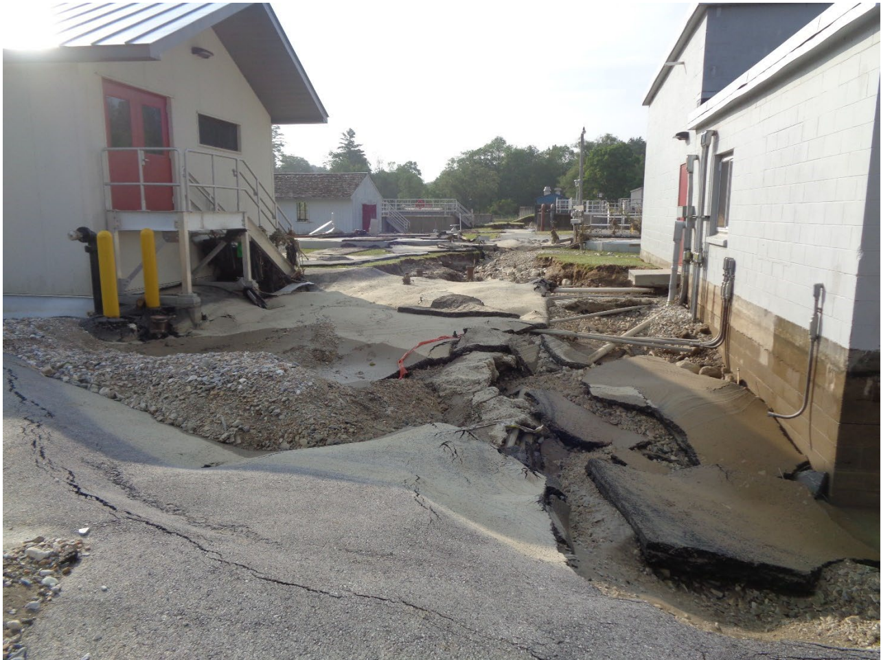
7 – Left Side: Influent Pump Station, Right Side Main Control Building. Displaced Asphalt Deposited, Extreme Scour, and Exposed Conduit and Piping (Photo courtesy of Aldrich and Elliot, PC)
