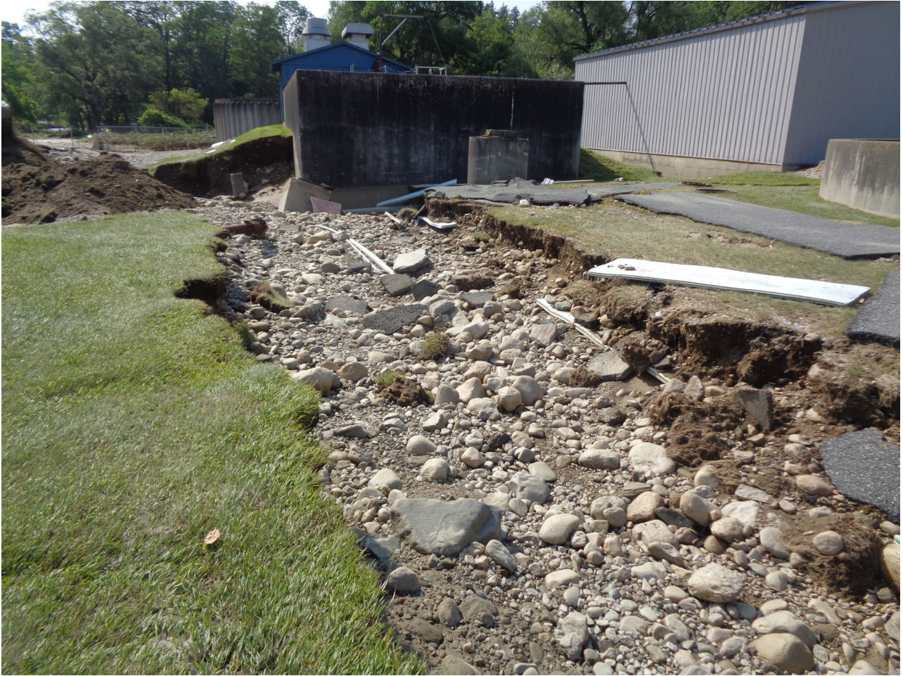
23- Aerobic Digester. Note Extreme Scour and Debris (Photo courtesy of Aldrich and Elliot, PC)
