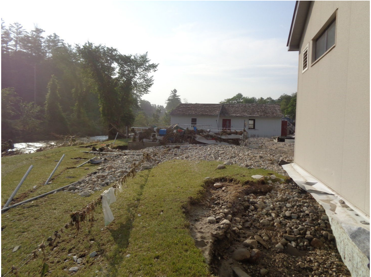
8 – Back of Influent Pump Station, Looking Towards Chlorine Contact Chamber. Note Extreme Scour and Damaged Site Fencing (Photo courtesy of Aldrich and Elliot, PC)
