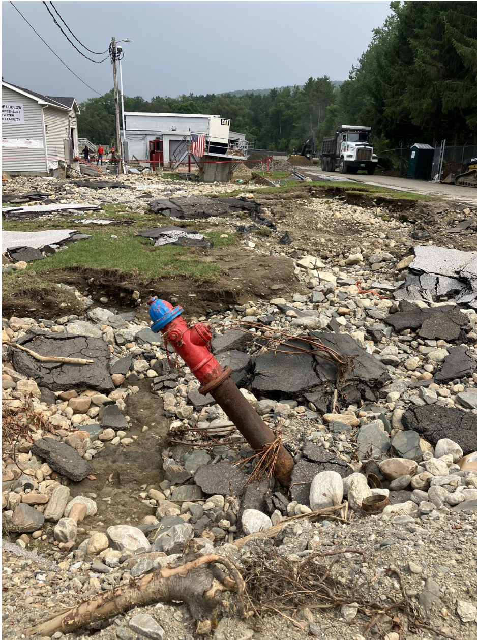
1 – Entrance to Ludlow WWTF Showing Extreme Scour and Asphalt Displacement
