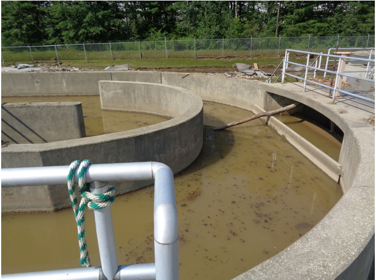
17 – West Oxidation Ditch Interior. Note Debris
