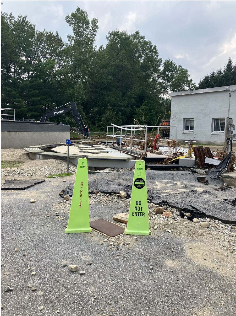
12 –Clarifier No. 2. In foreground, Clarifier No. 3 in Background. Note Debris and Extreme Scour
