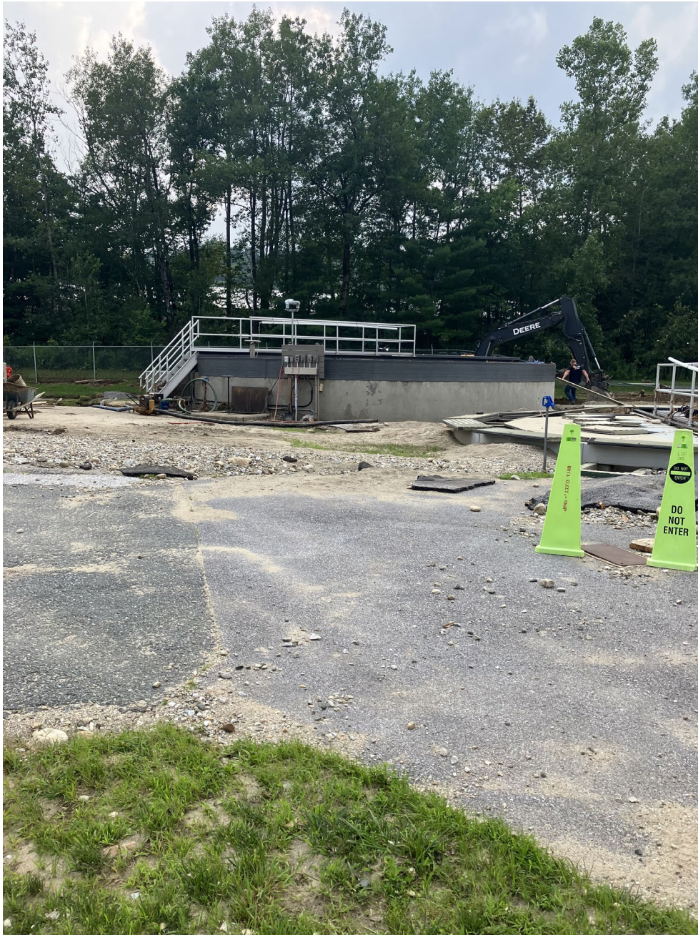
13 –Clarifier No. 3. Note Debris and Extreme Scour
