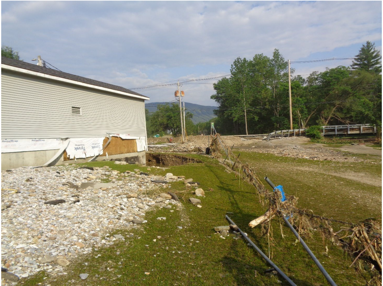
5 – Left Side: Headworks Building, Looking Back Towards Entrance. Damage to Exterior of Building and Extreme Scour and Site Fence Damage (Photo courtesy of Aldrich and Elliot, PC)
