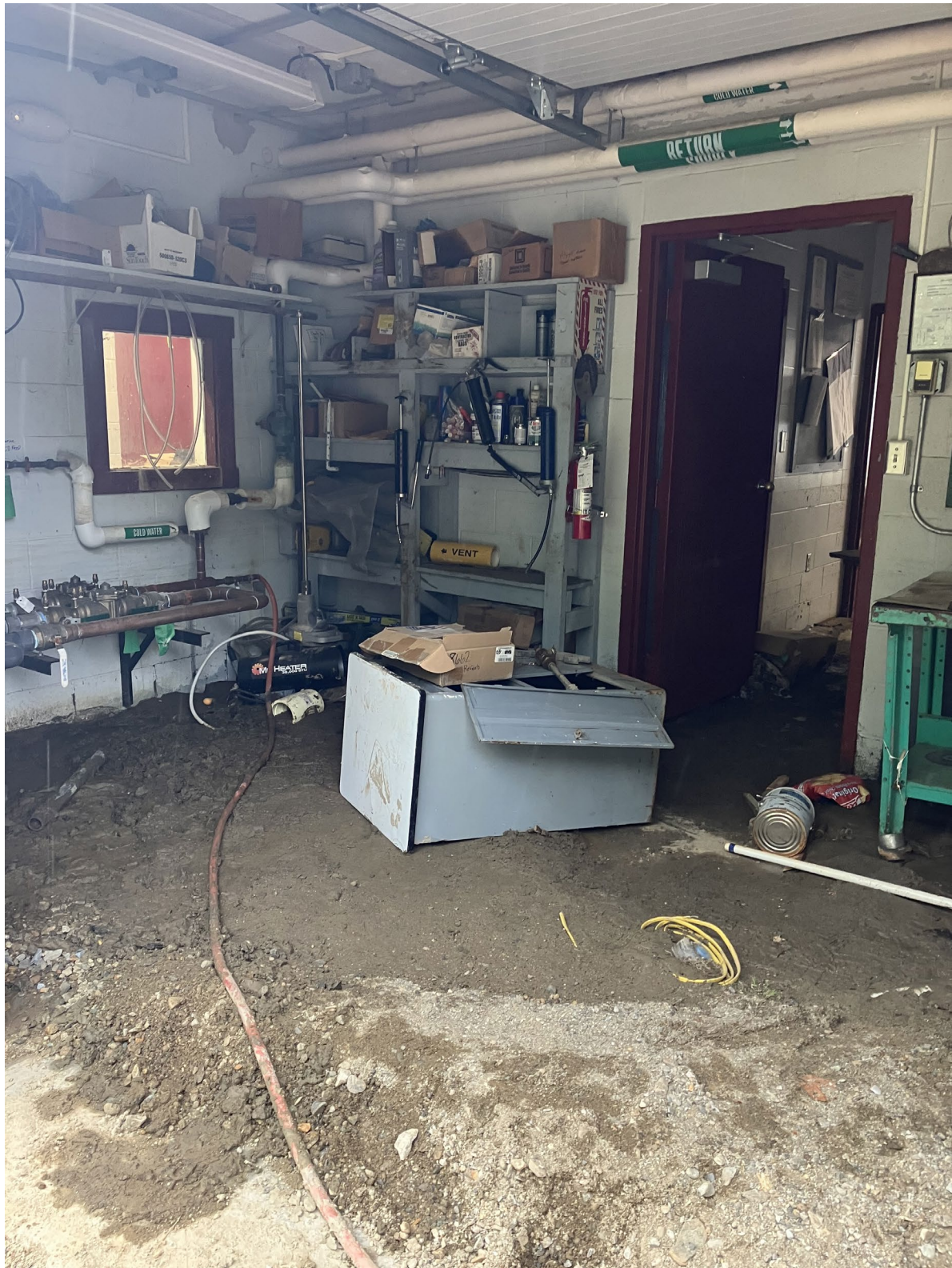
29- Main Control Building Maintenance Room.
