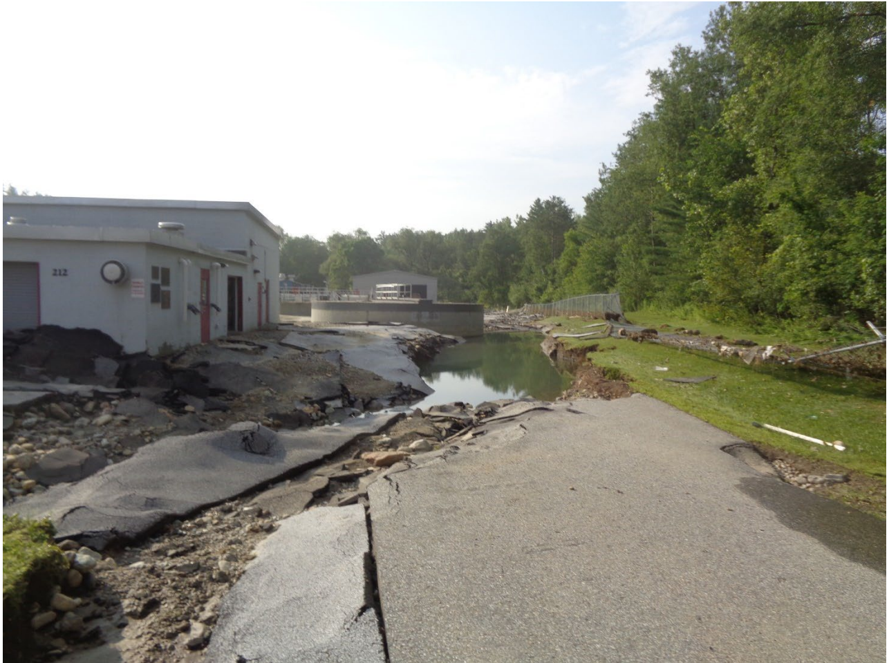
2 – Entrance to Ludlow WWTF Showing Extreme Scour and Asphalt Displacement, No. 3 Secondary Clarifier in the Background (Photo courtesy of Aldrich and Elliot, PC)
