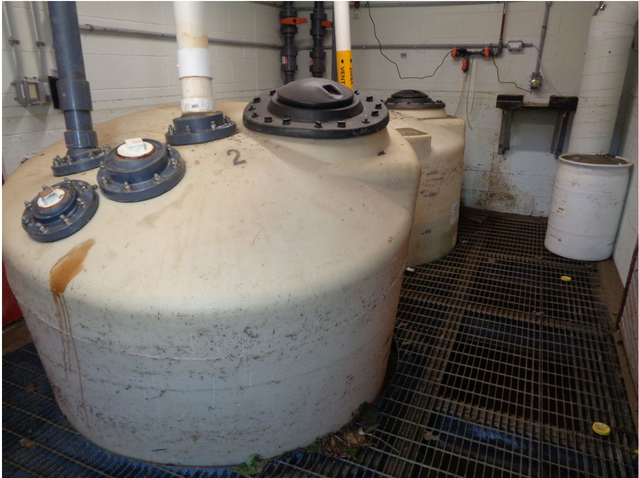
27- Main Control Building Bisulfite Tanks. Note High Water Mark at Approximately 4 Feet. (Photo courtesy of Aldrich and Elliot, PC)
