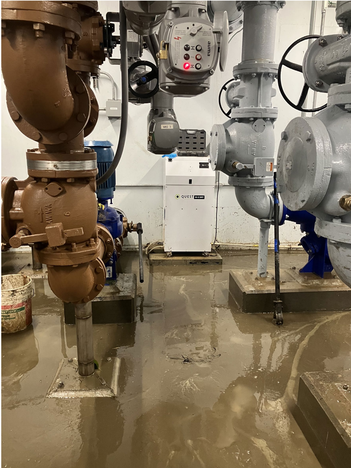
10 – Basement Area of Influent Pump Station Showing Influent Pumps, Sludge Pumps and Dehumidifier, High Water Mark at approximately 18”.
