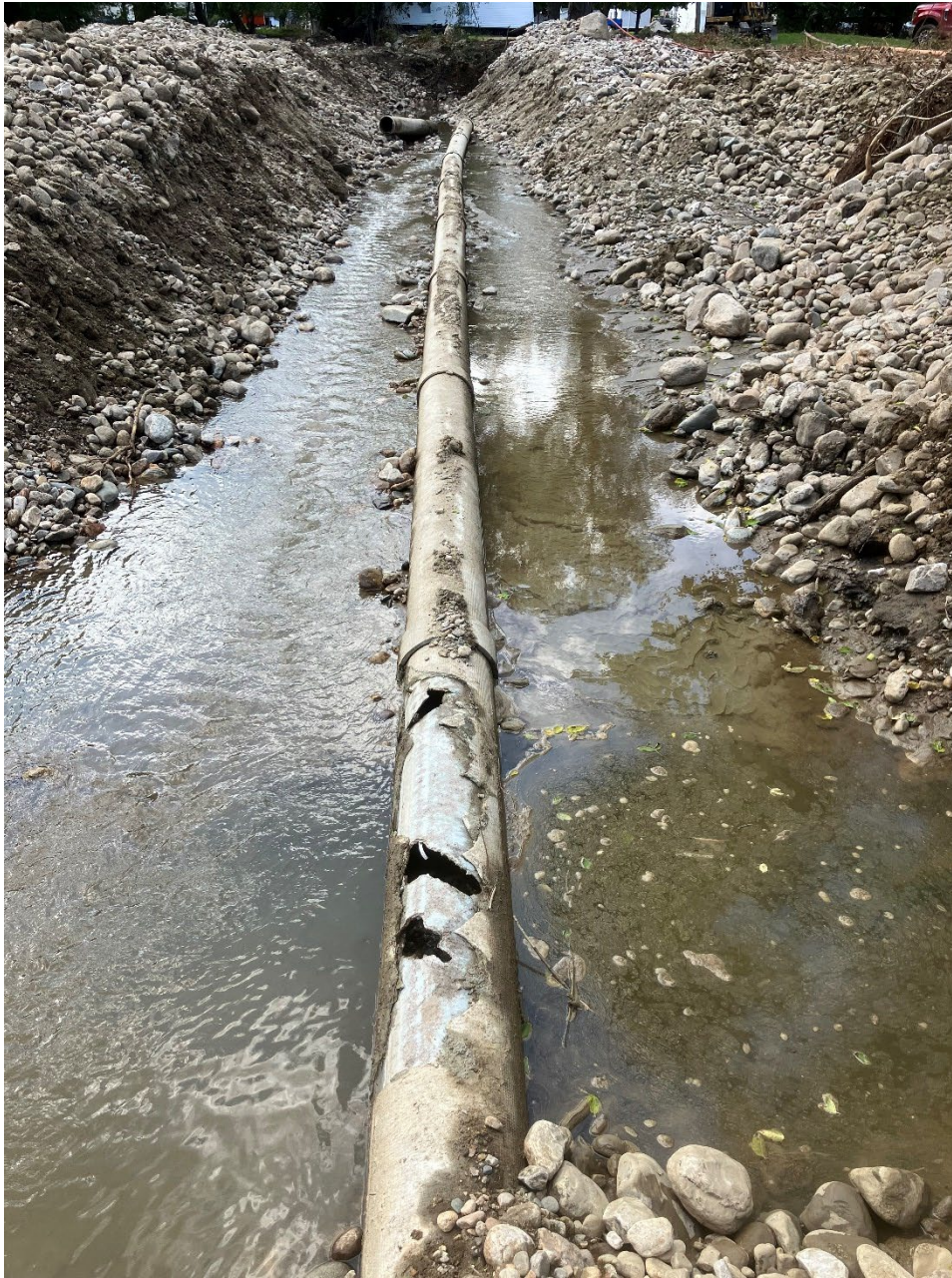
30- 15" AC Sewer Main Along Black River (Photo courtesy of Chief operator Joe Gaudiana)
