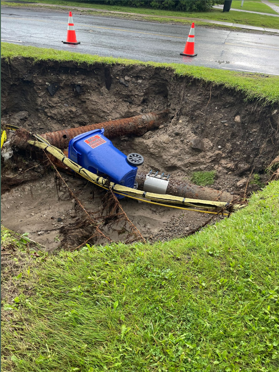
Figure 1: Sinkhole at Maverick Gas Station
