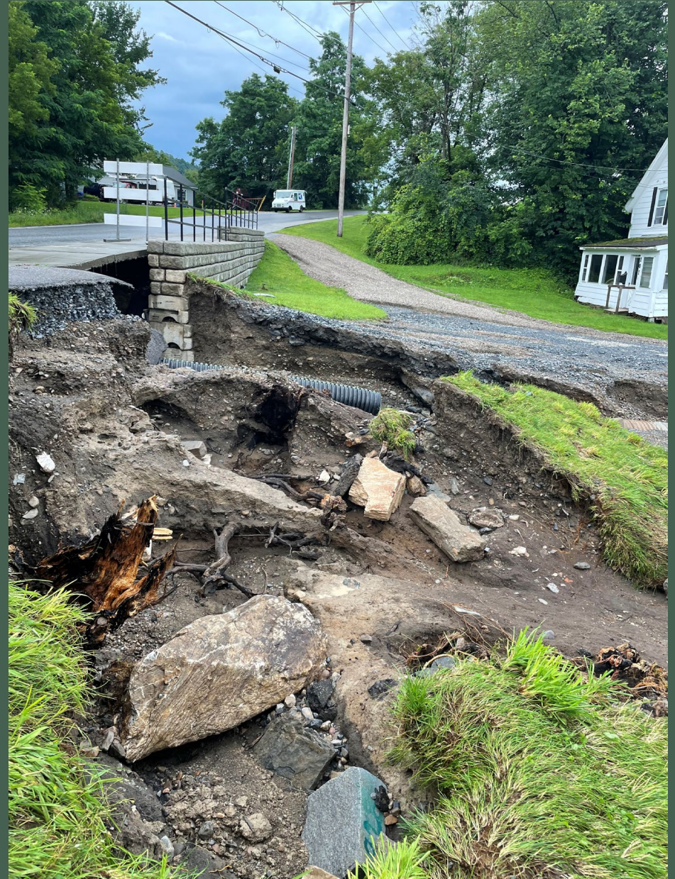
Figure 2: Seymour St- Culvert Failure
