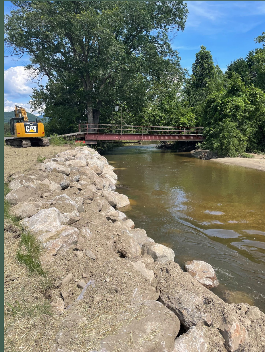
Three Mile Bridge Rd- significant scour
