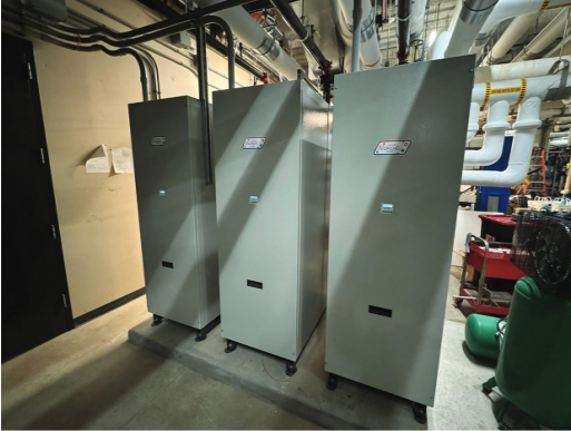
Three water to water heat pumps
