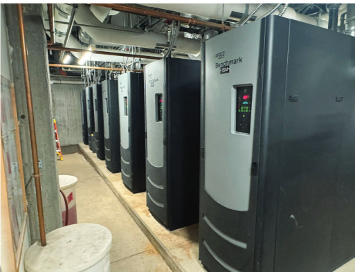
Seven of the propane boilers the electric boiler takes the place of during operation
