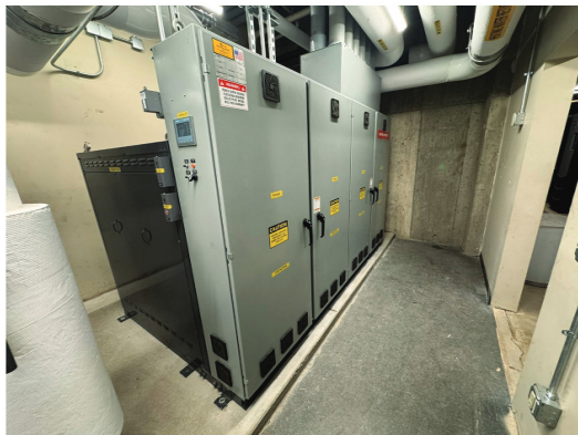
Boiler and electric cabinet
