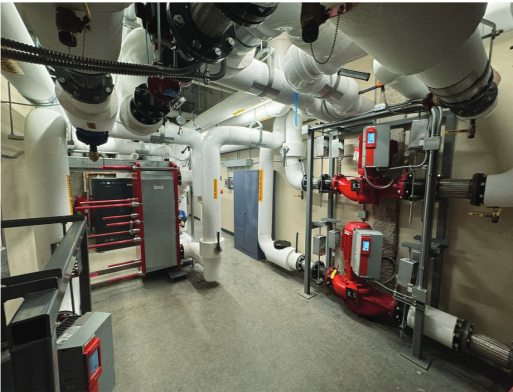
Electric boiler room
