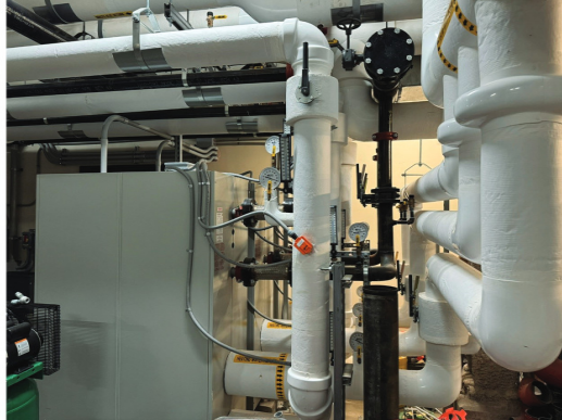
Heat pumps and associated piping
