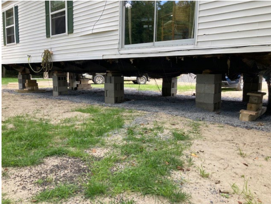
Figure 4: A home in Black River Mobile Court in Ludlow, impacted by water intrusion, gutted to avoid mold growth and being raised on its foundation to minimize future flooding damage.
