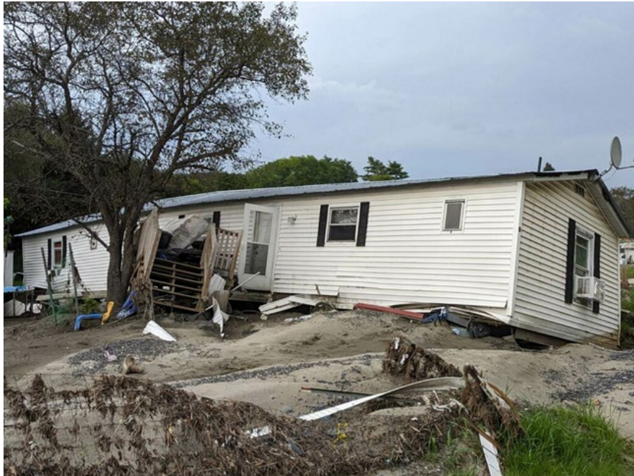
Figure 2: Home in River Run Mobile Home Park in Berlin showing extent of the damage. (Photo by JoEllen Calderara)
