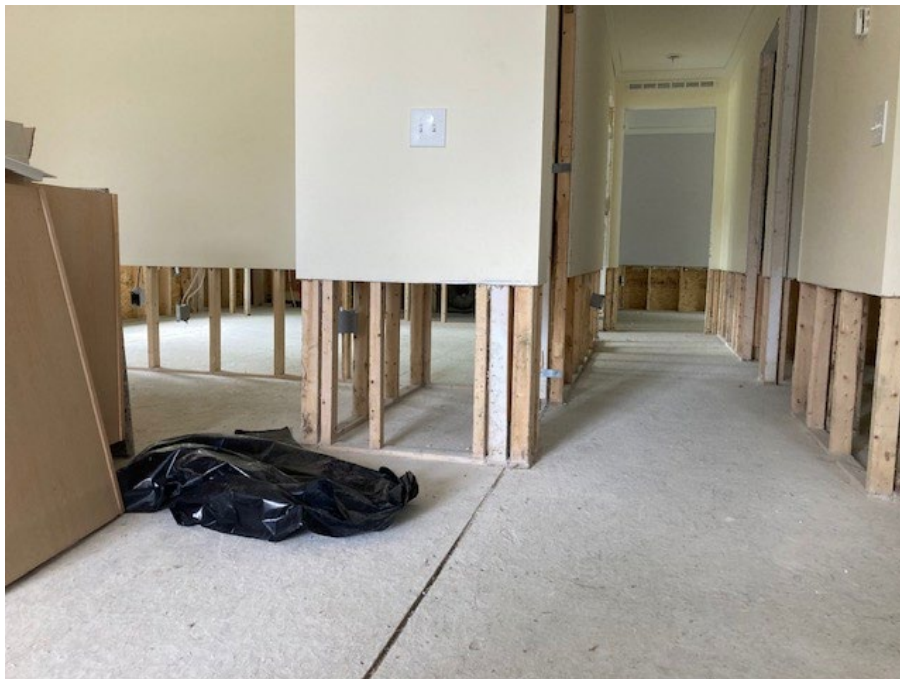
Figure 3: The interior of a home in Highland Heights MHP in Johnson, gutted to prevent further water and mold damage.
