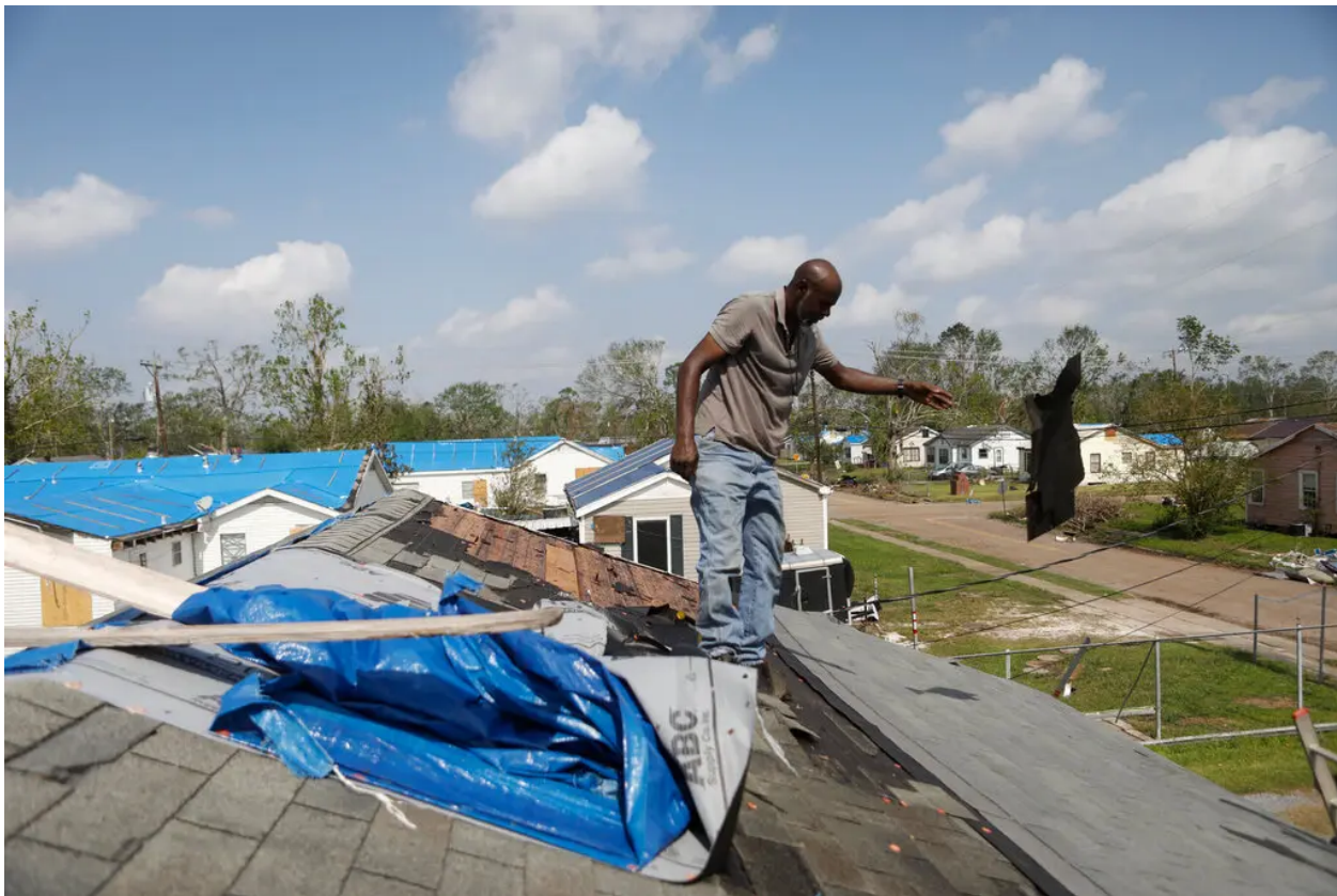
Gary Hanney worked on repairing his brother's roof in Lake Charles after it was damaged by Hurricane Laura. Octavio Jones for The New York Times
