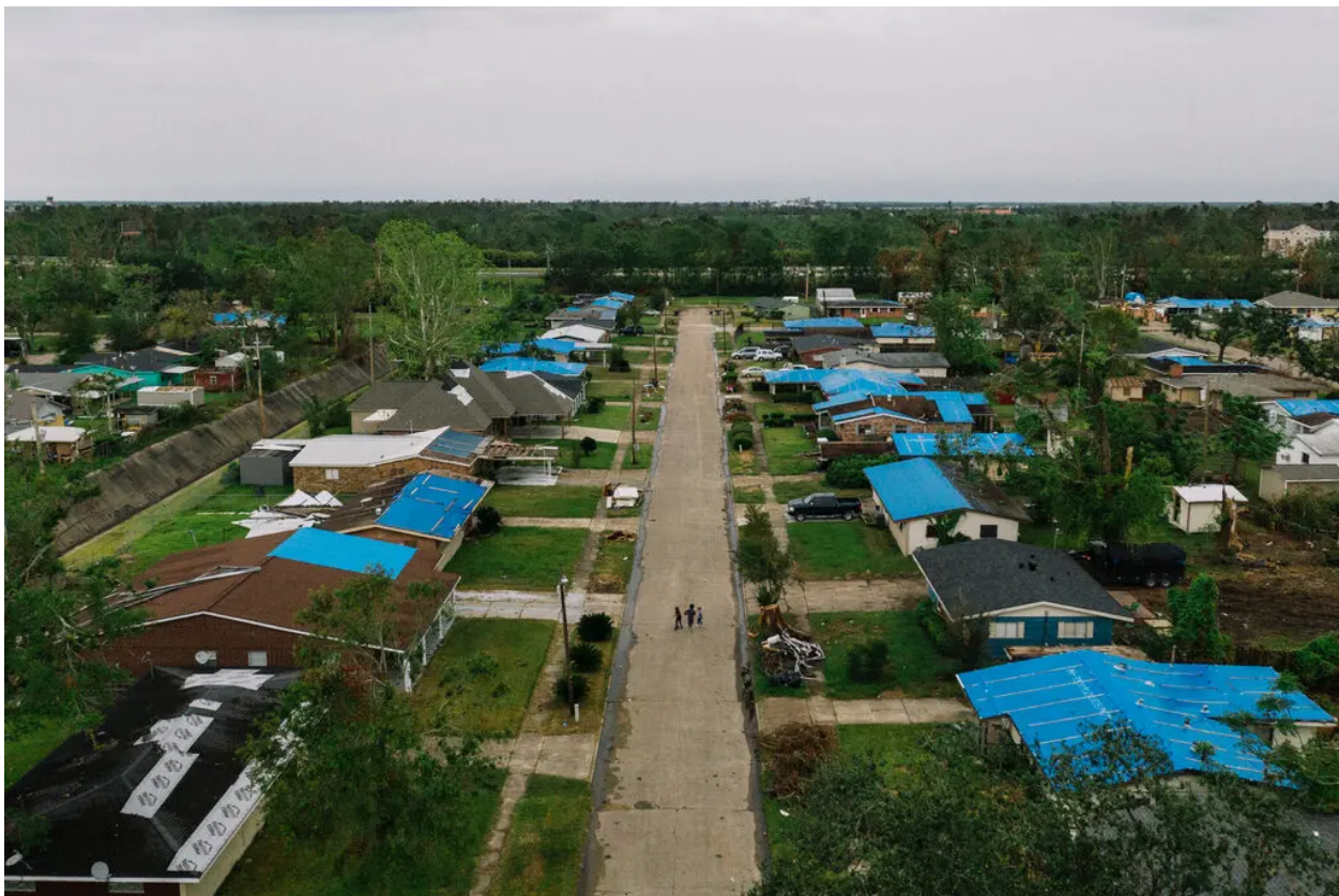
Homes in Lake Charles, temporarily fitted with tarps to cover damaged roofs, braced for Hurricane Delta, which arrived just six weeks after Hurricane Laura in 2020. William Widmer for The New York Times
