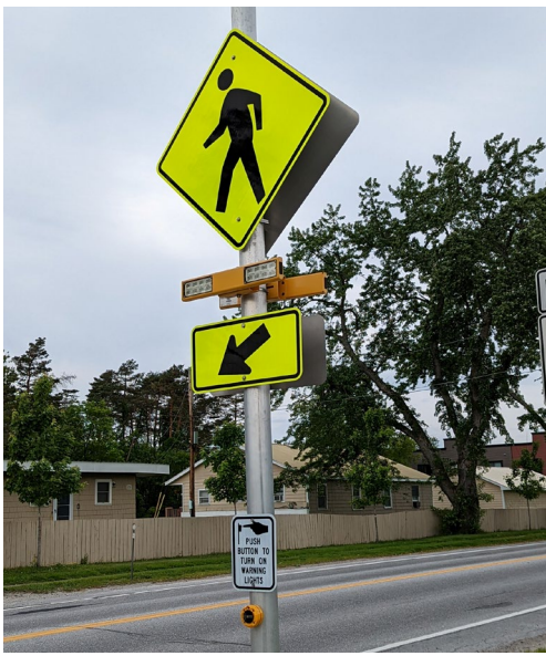
Rectangular rapid flashing beacons (RRFB)
