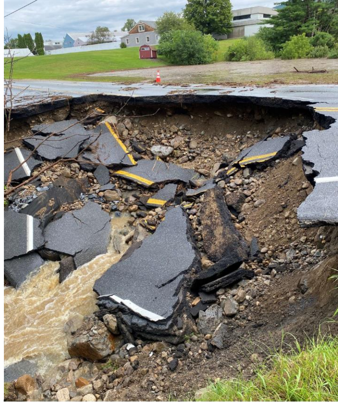
Dow Pond Dam, Middlebury, SIGN Hazard
