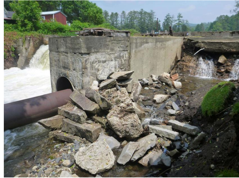
East Calais Mill Dam, East Calais, SIGN Hazard
