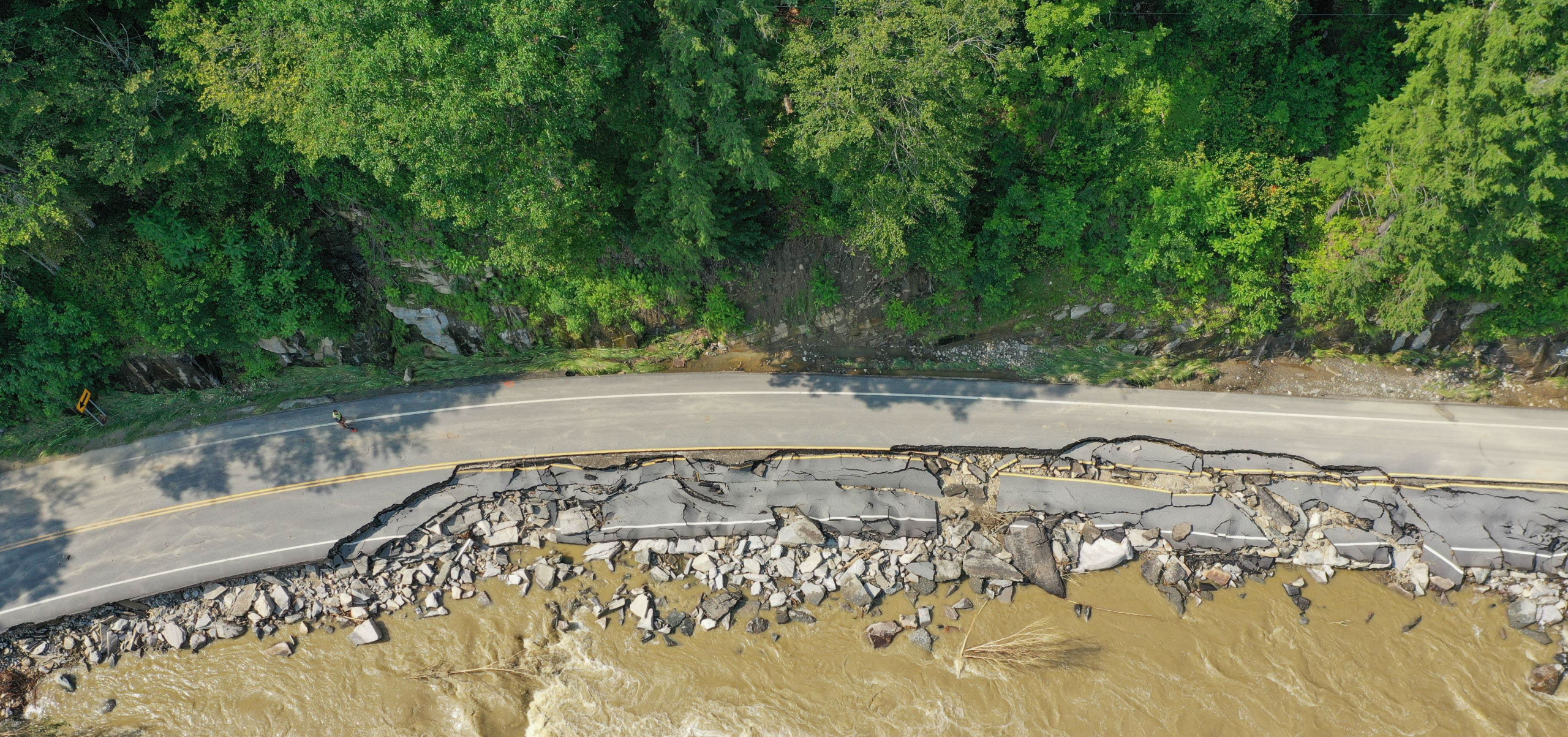
Cavendish VT106 Washout
