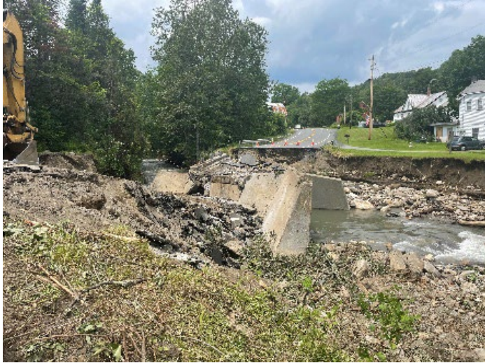
Vershire Bridge 13 on VT 113 Before and After (Installation of a Temporary Bridge)
