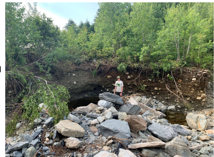
Gale Meadows Dam Aux. S/W damage and temp. repair
