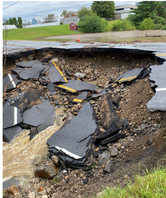
Dow Pond Dam, Middlebury, SIGN Hazard
