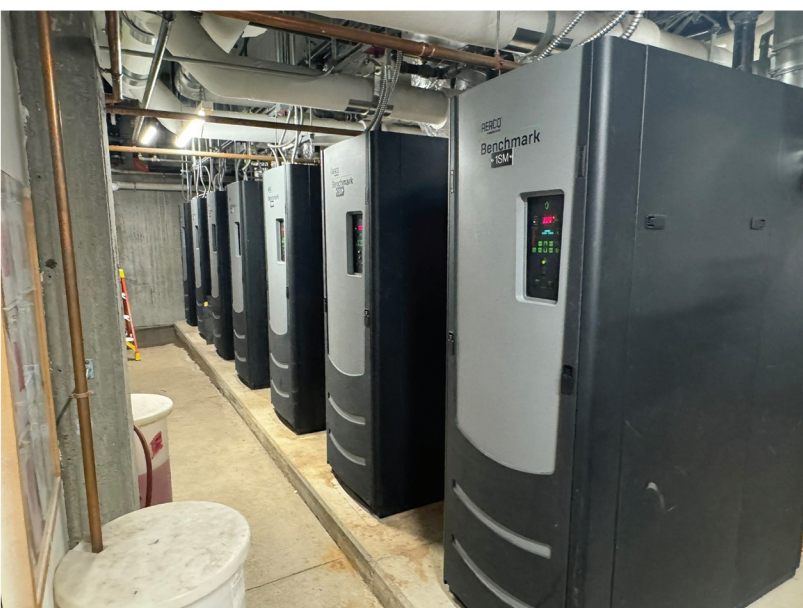
Seven of the propane boilers the electric boiler takes the place of during operation
