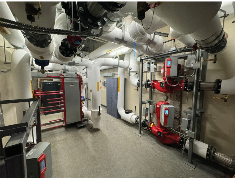
Electric boiler room
