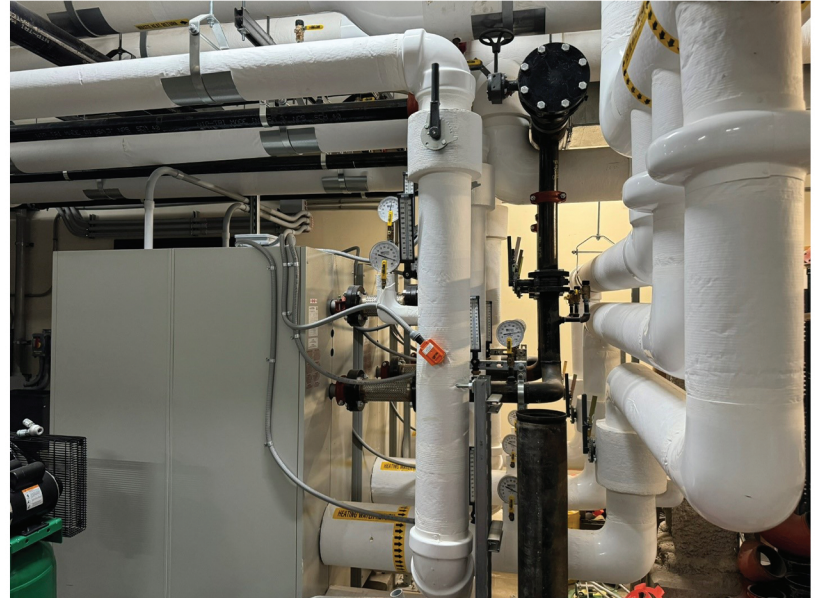
Heat pumps and associated piping
