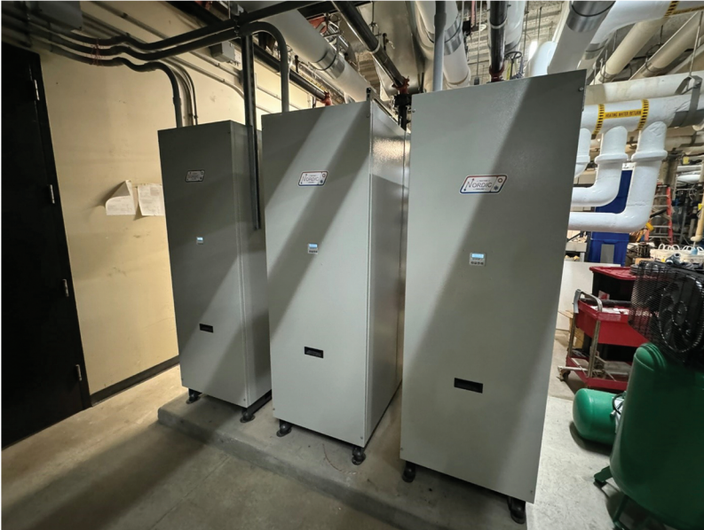
Three water to water heat pumps
