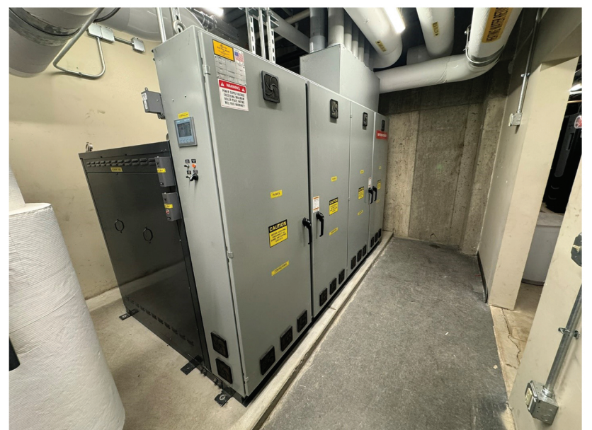
Boiler and electric cabinet
