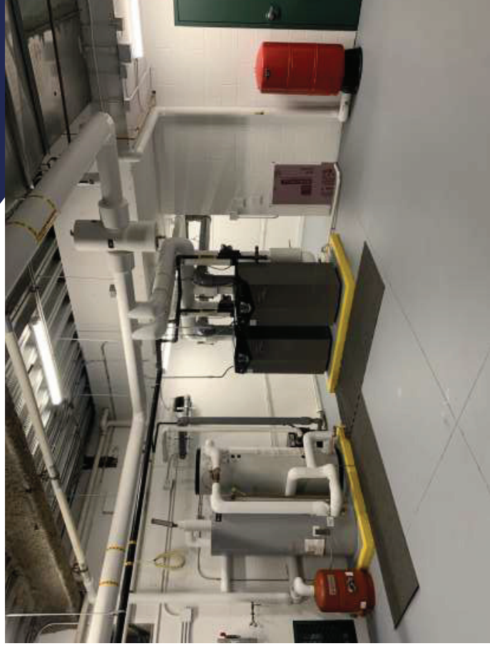
Franklin Elementary School, VT – 2022 - Oil to LP w/ Condensing Boilers
