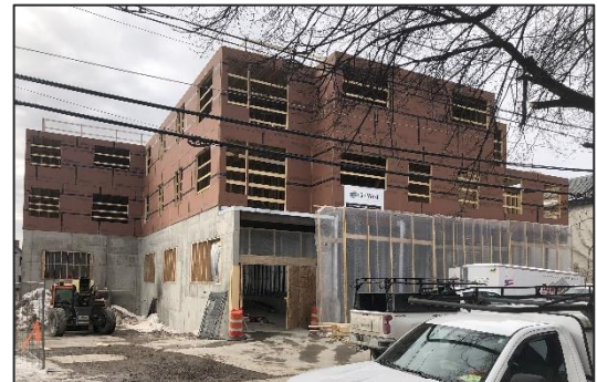
Development of 48 rental units under construction located at 151-157 South Champlain street. Photo provided by the City of Burlington.
