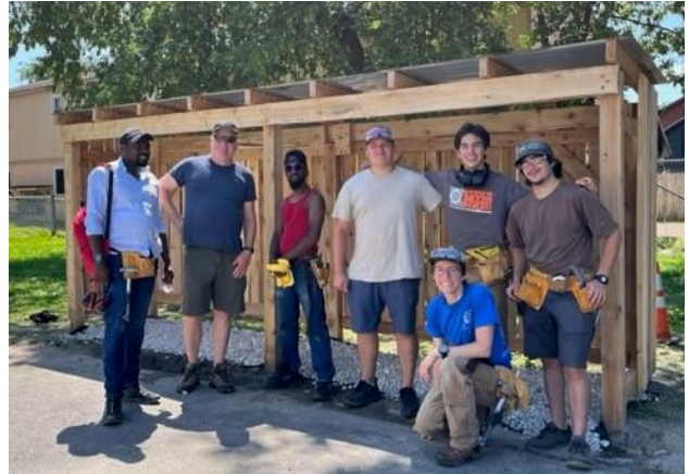
Construction 101 group from ReSOURCE completing an overhead structure for Champlain Housing Trust where trash and recycling cans will now be stored
