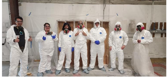
The ReSOURCE weatherization training intensive participants suited up for spray foam training. This course occurred in Bennington, VT.
