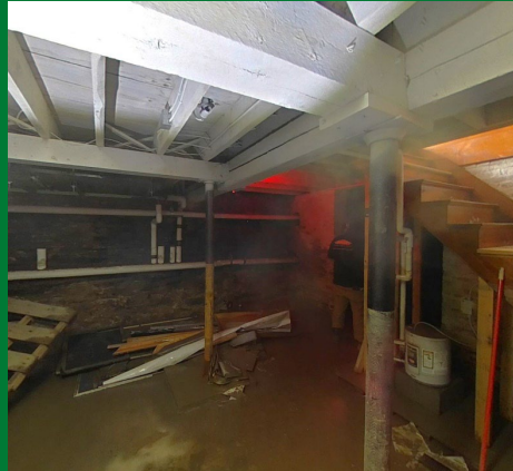
Group 1: South side of street, basement impacted
