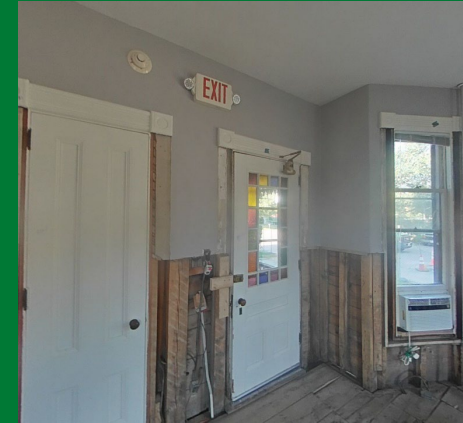
Group 2: South side of street, basement and first floor impacted
