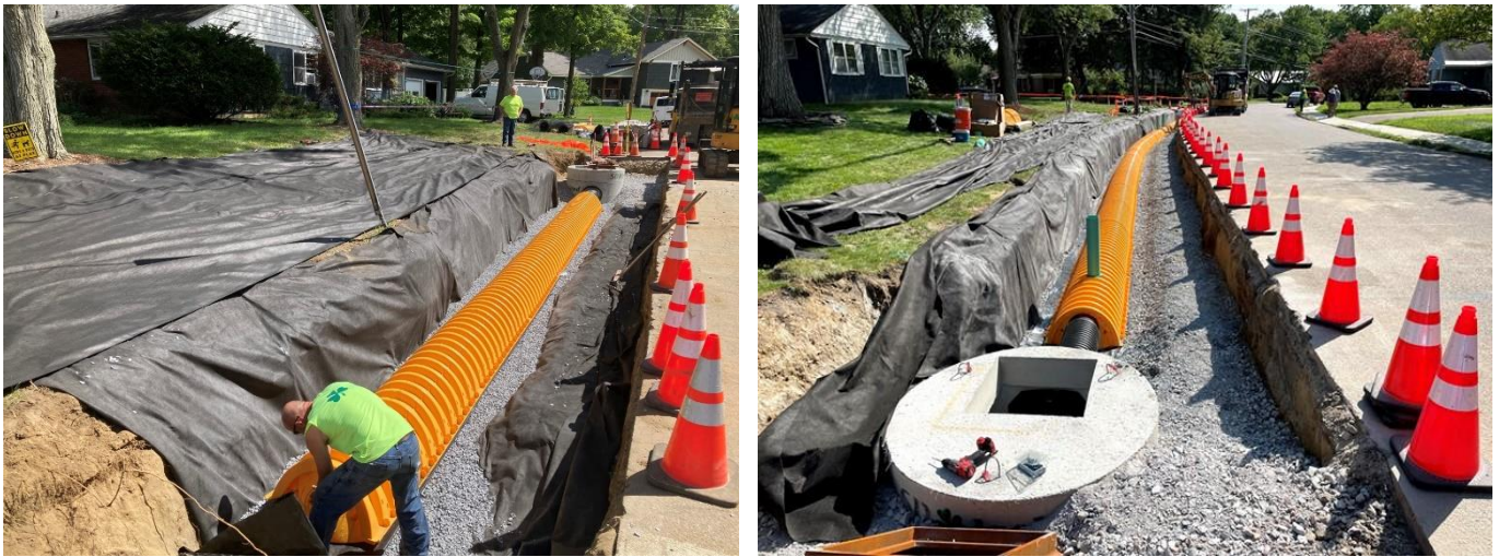
Figure 19: Phosphorus reduction on developed land is required to implement the Lake Champlain TMDL. This project contributes to that reduction by providing stormwater treatment for untreated developed lands in a Burlington neighborhood via Green Stormwater Infrastructure (GSI). The image depicts installation of a stormwater infiltration chamber, a GSI technique. Runoff can fill the large yellow structure, then seep slowly into the crushed rock base and soils below. This infrastructure reduces polluted runoff and high stormflows from developed lands that drain into combined sewer systems and contribute to combined sewer overflows. This project was funded through Lake Champlain Basin Program dollars administered by the Department of Environmental Conservation.
